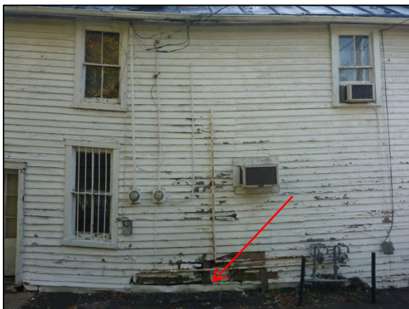
View of left side of house at obvious foundation failure
