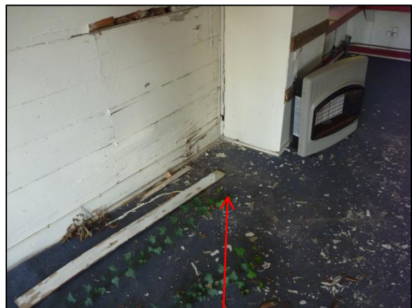
View of interior at chimney showing sagging floor
