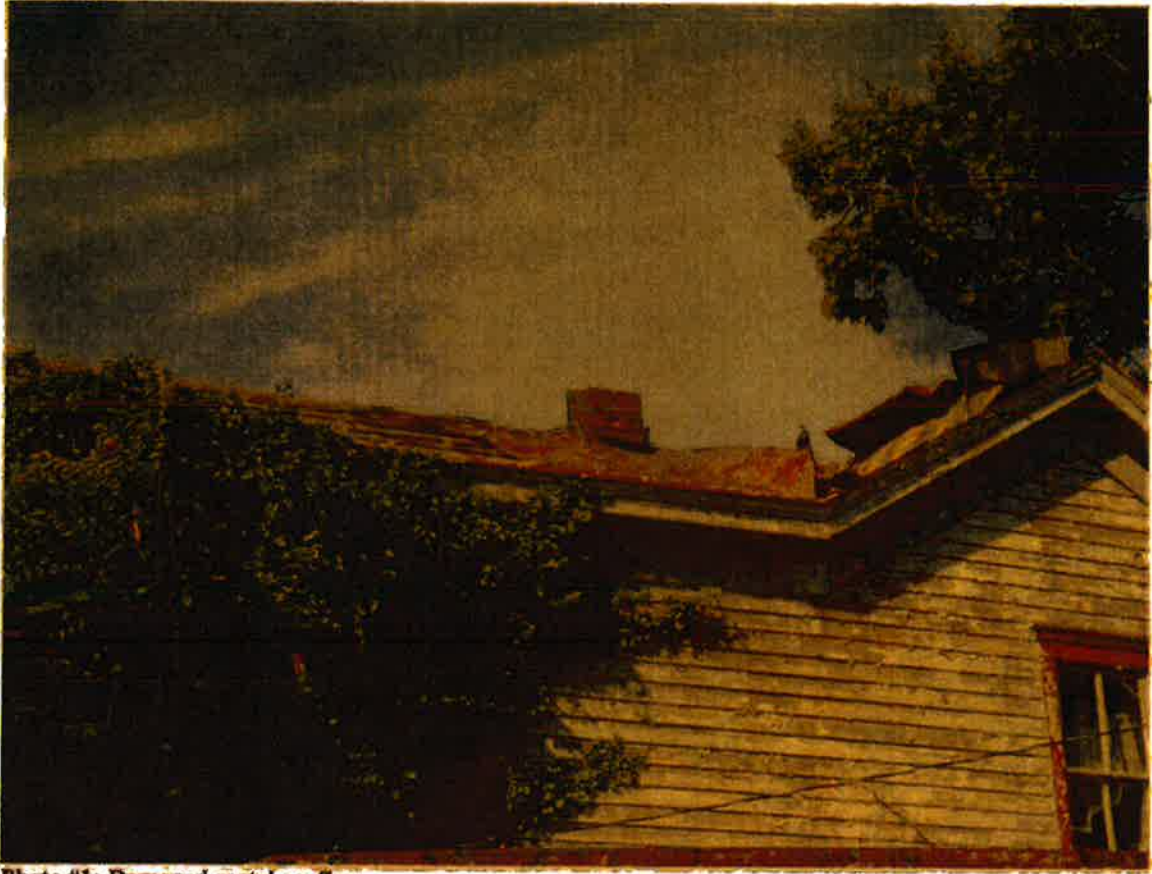
Photo #1: Damaged metal roofing
