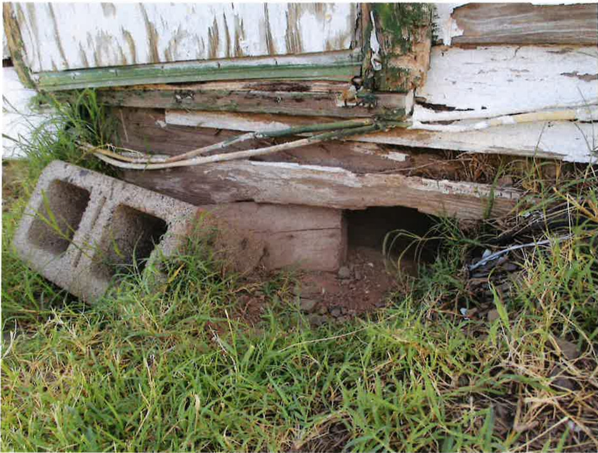
Photo #2: Additional animal holes with CMU/wood shoring present below the sill.
