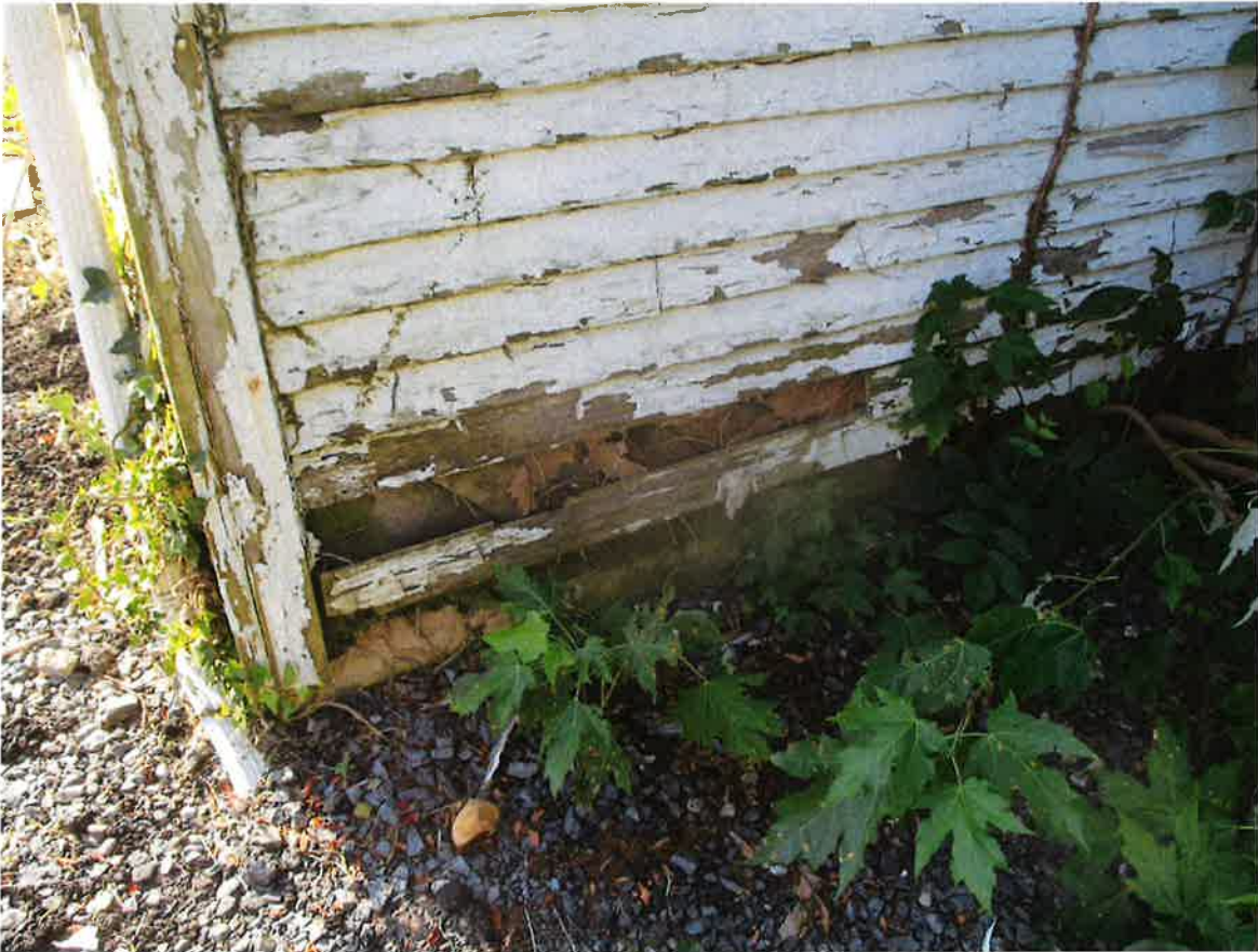
Photo #8: Rotted and missing sheathing boards.
