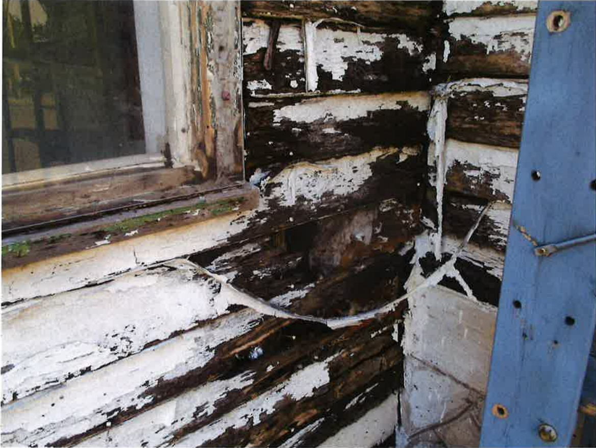
Photo #9: Severely rotted wall sheathing with rotted wall studs beyond.
