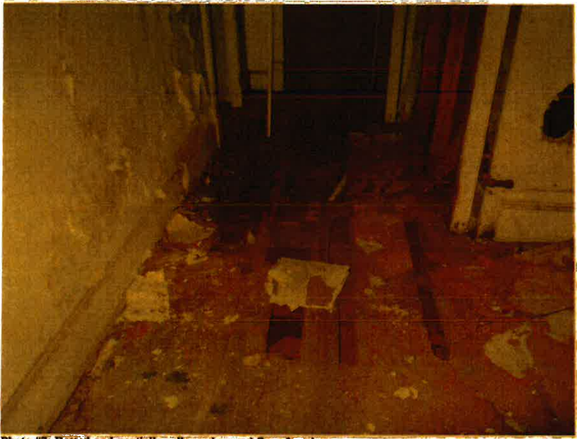
Photo #7: Rotted and partially collapsed second floor framing.
