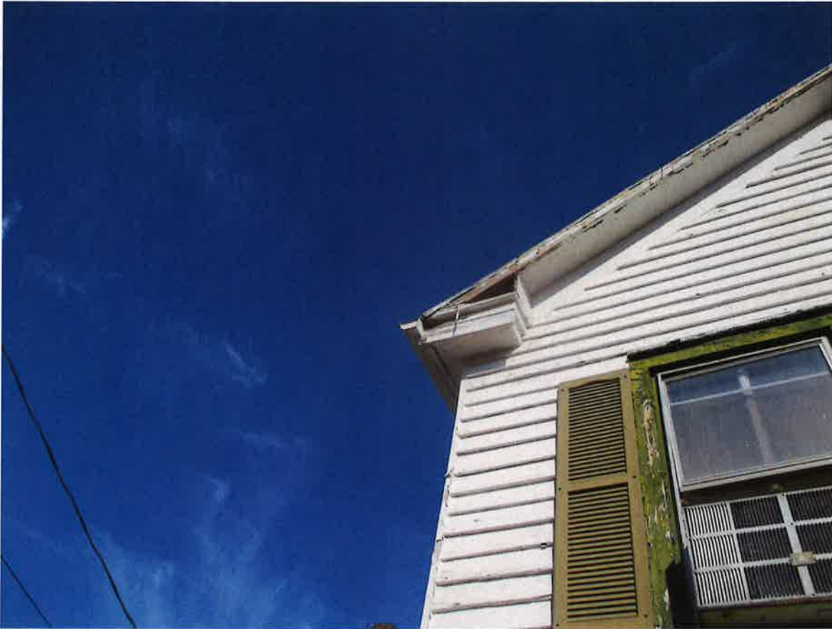
Photo #8: Missing fascia board at eave of roof.
