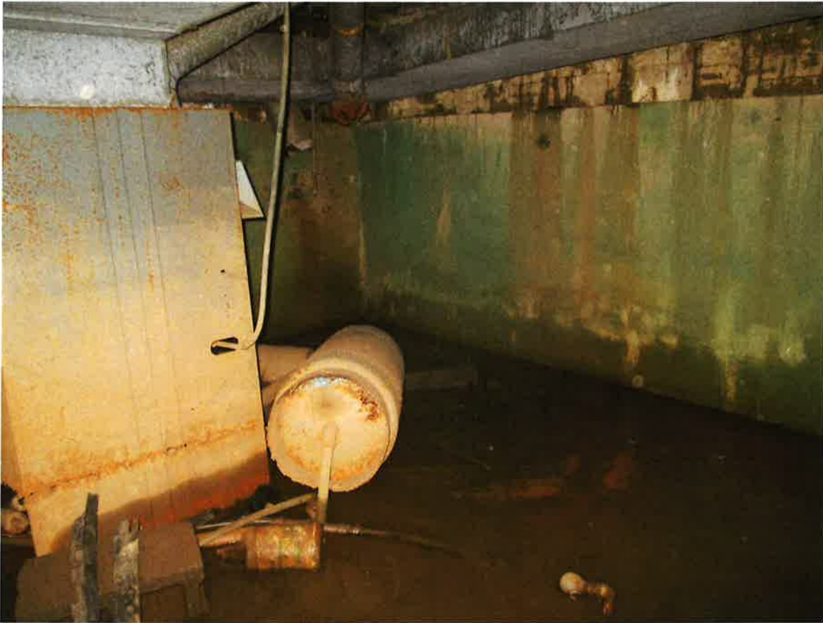
Photo #11: Standing water throughout basement level.
