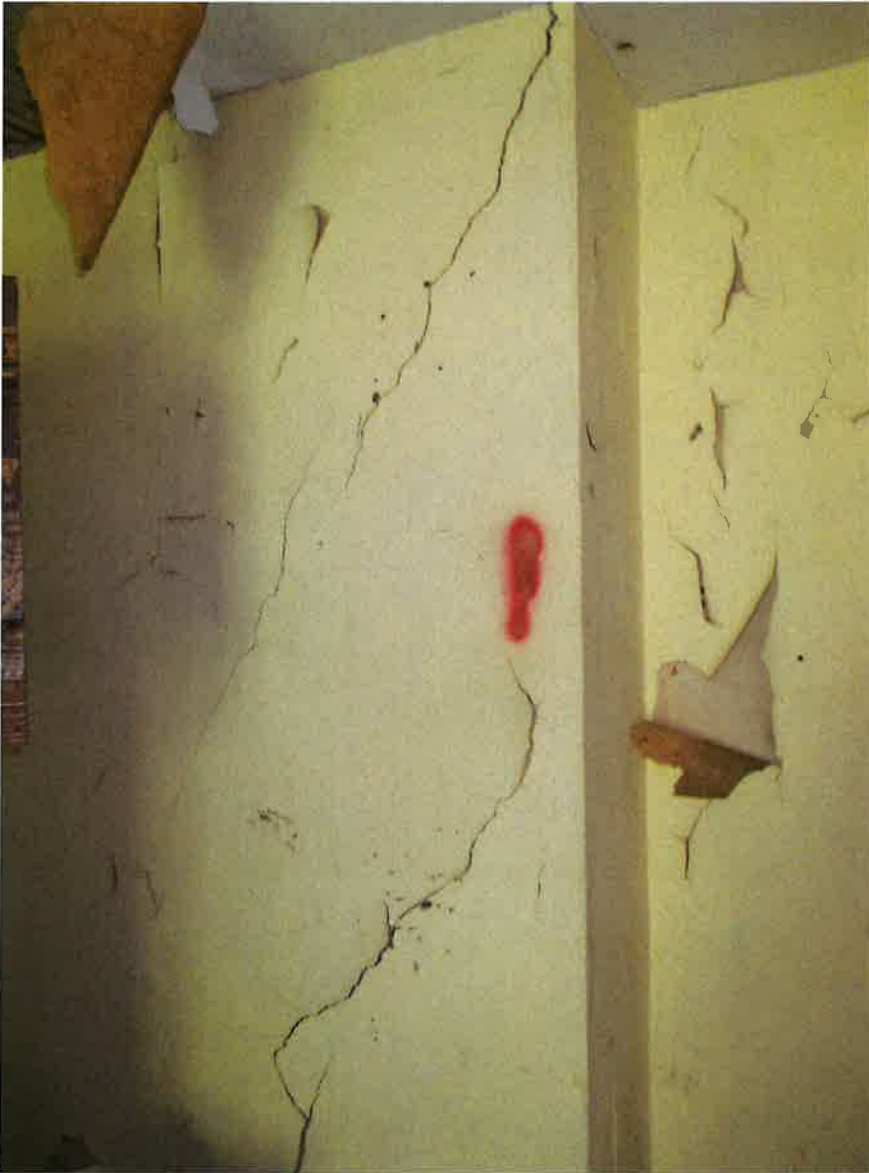
Photo #10: Diagonal plaster cracks at interior of chimney.
