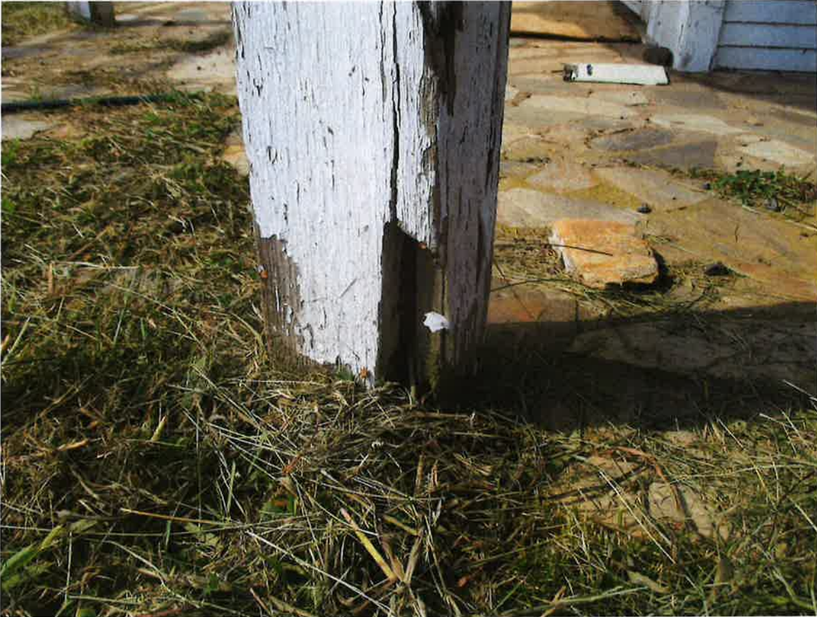
Photo #3: Rot at base of porch post.
