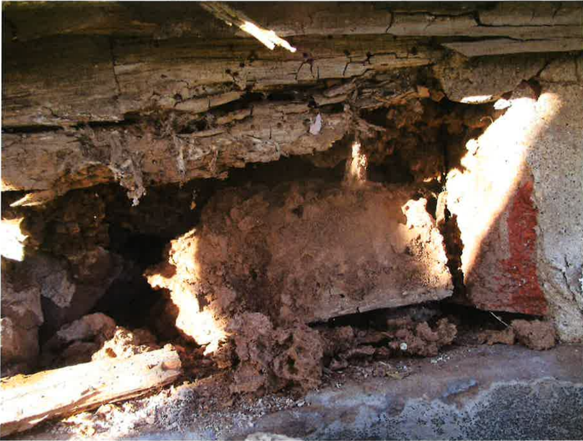
Photo #3: Severely rotted and deteriorated wood sill.
