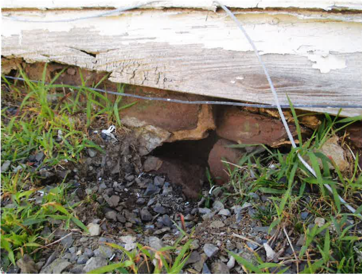
Photo #12: Large voids are present at the base of the stone foundation wall.
