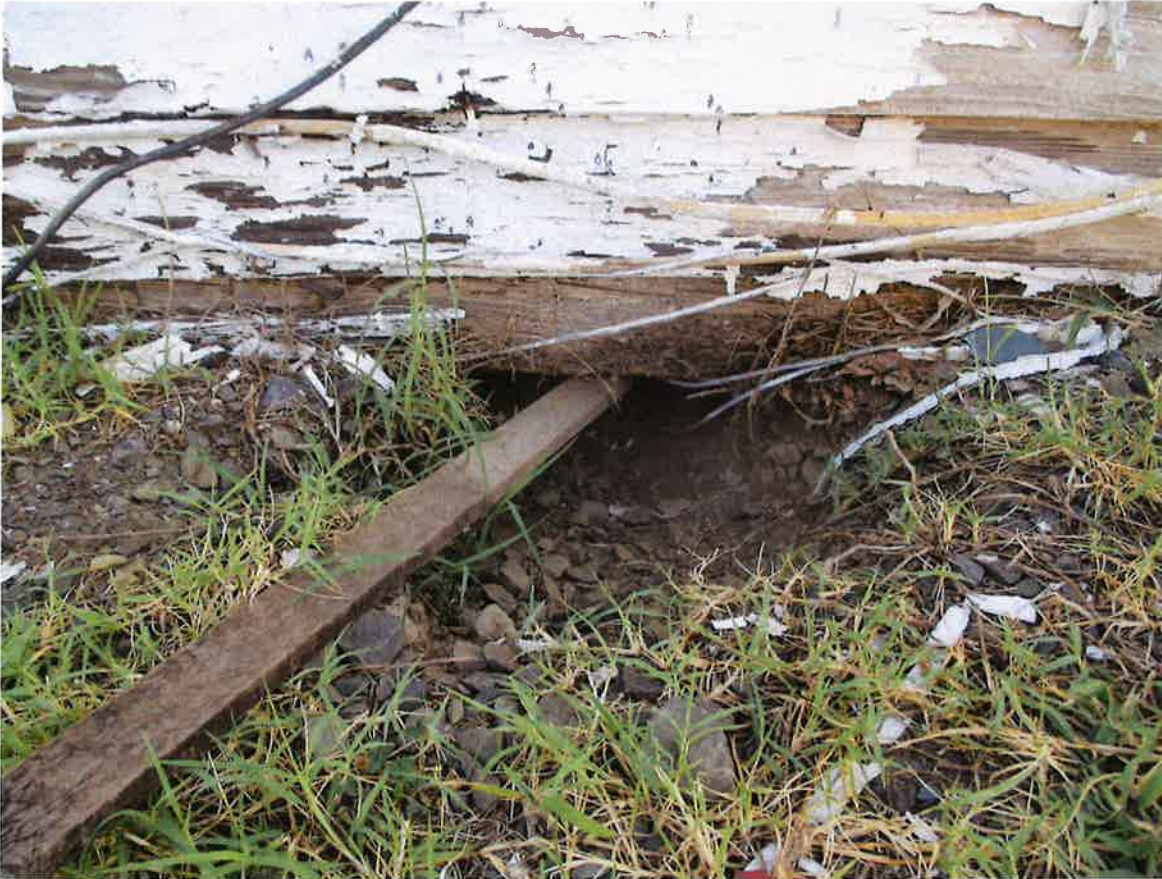
Photo #1: Animal hole undermining existing wood sill plate
