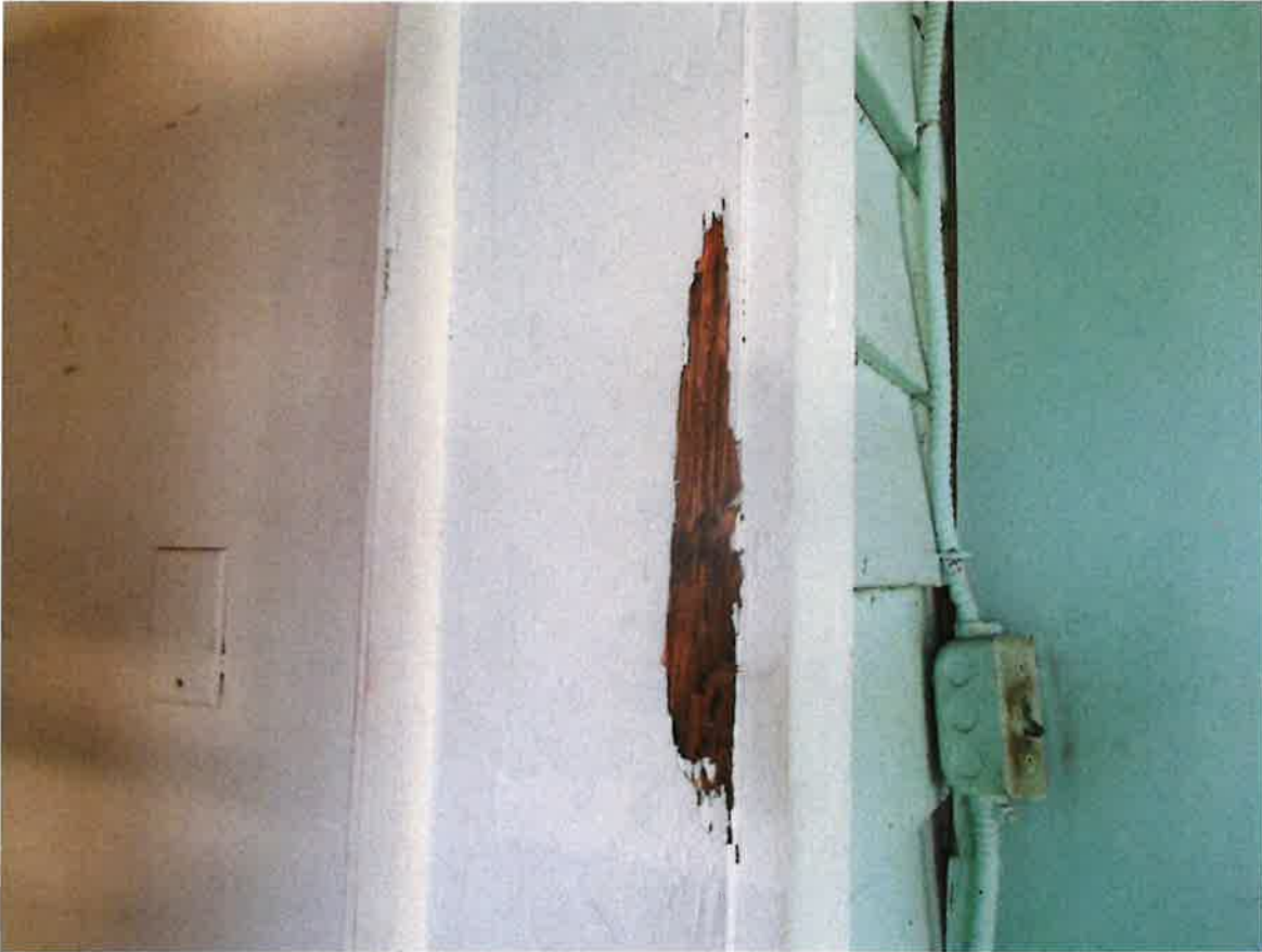
Photo #7: Termite damage at jamb of wall opening.
