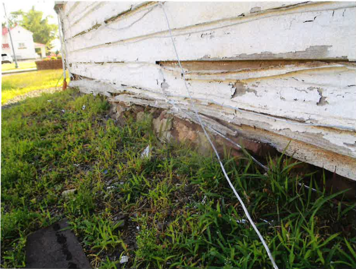
Photo #11: Base of siding board has rotted exposed wood sill plate to the exterior.
