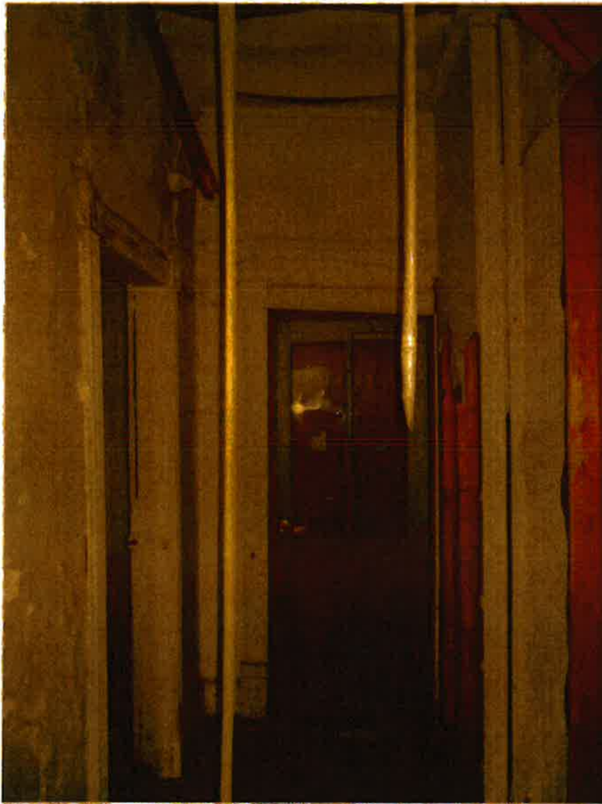
Photo #8: Severe sag at first floor door frame adjacent to bearing wall.
