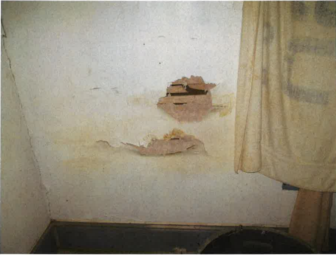
Photo #12: Plaster damage on face of wall.
