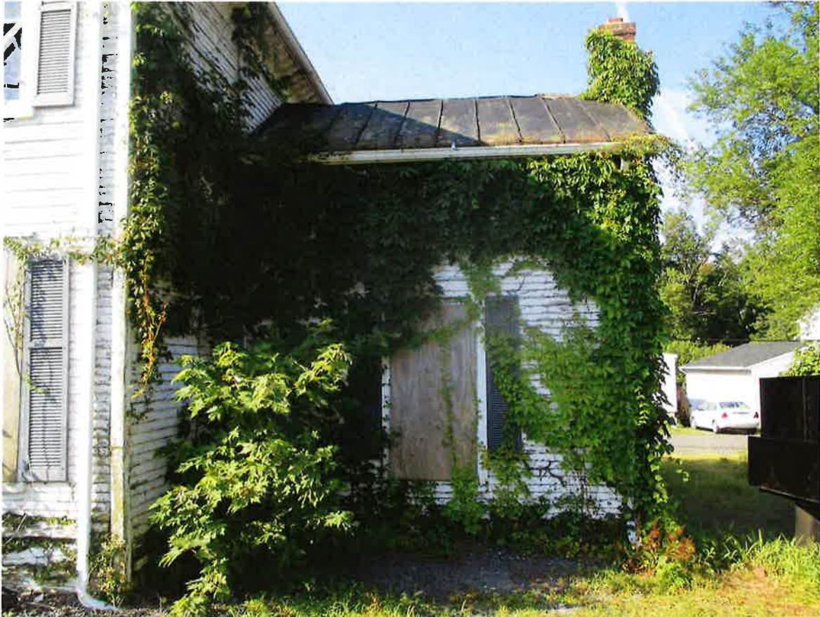
Photo #6: Vines over-growing rear 1-story portion of house.
