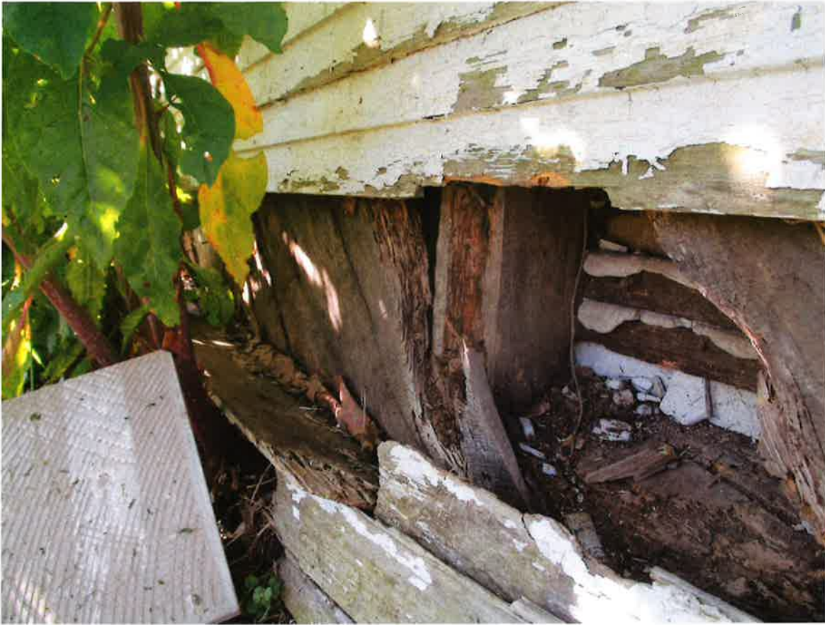
Photo #5: Exterior exposed and rotted wood studs, diagonal brace and sill plate.
