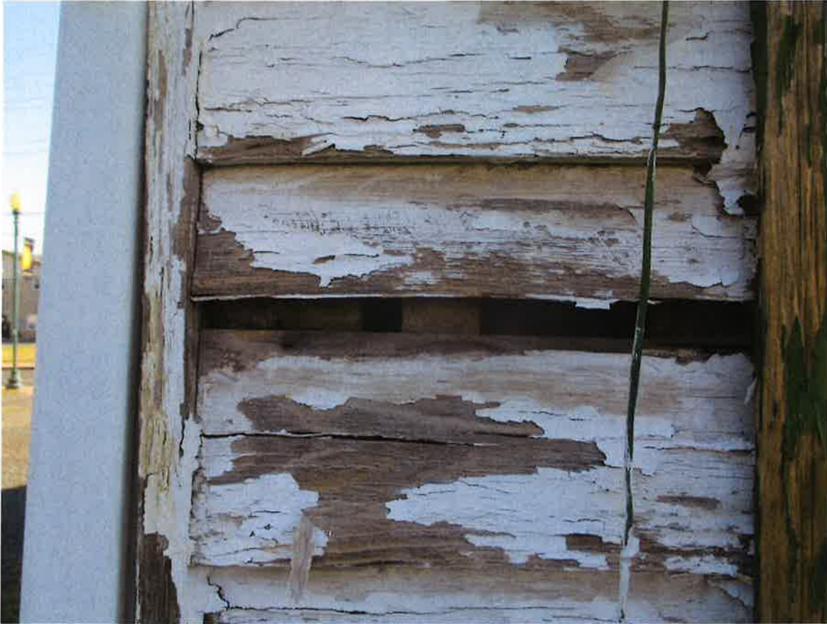
Photo #10: Void present between rotted siding boards.
