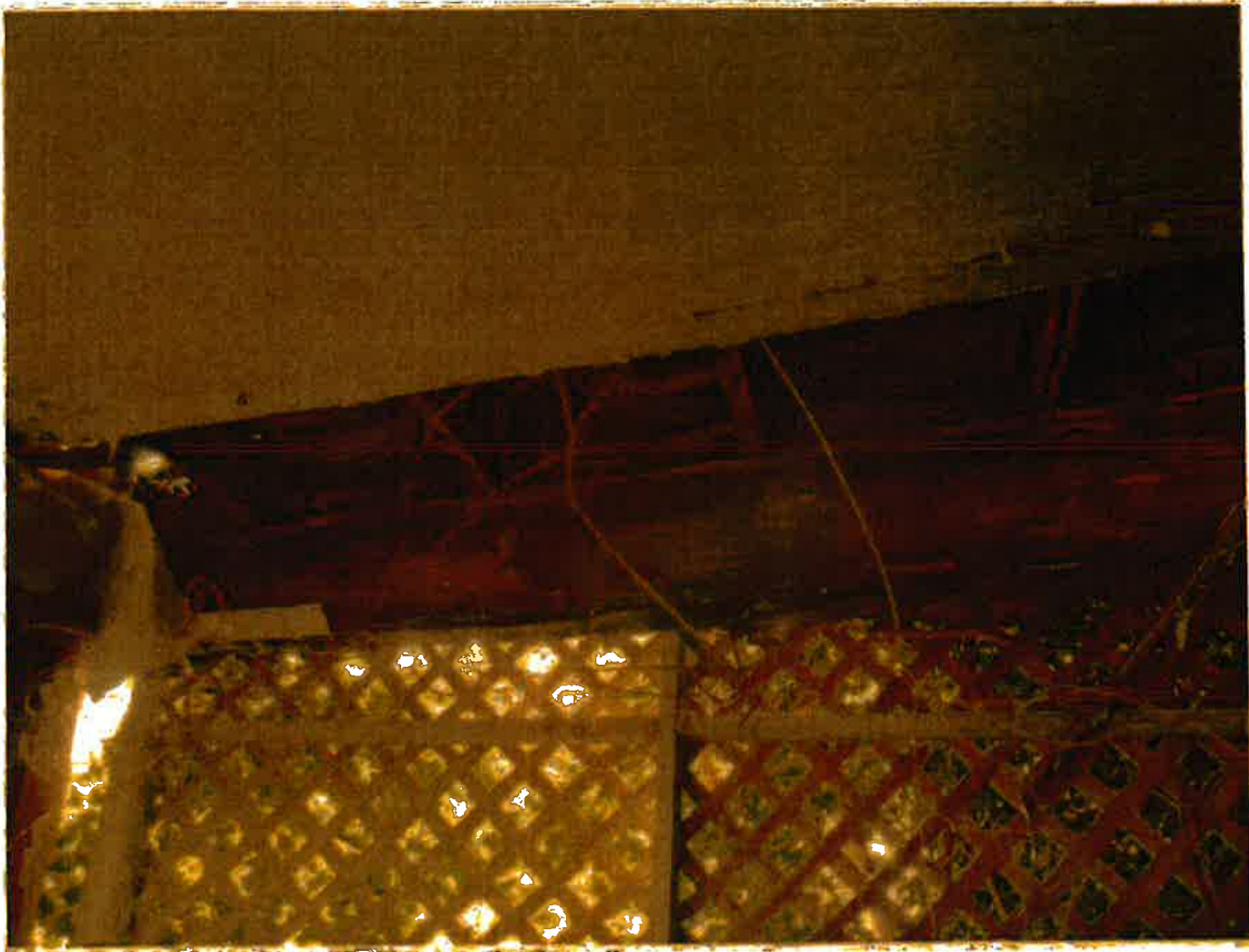
Photo #6: Rotted porch spandrel beam and rafter tails.
