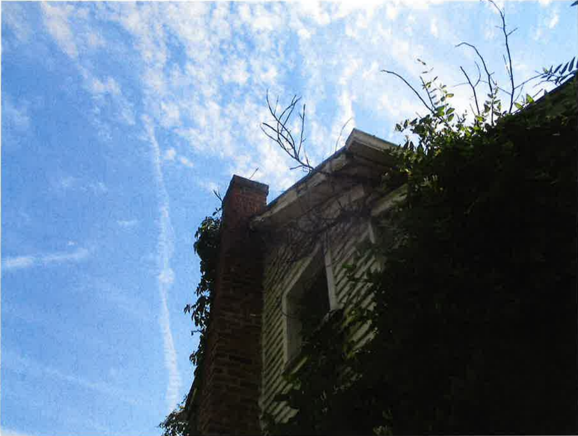
Photo #7: Rotted rake board.
