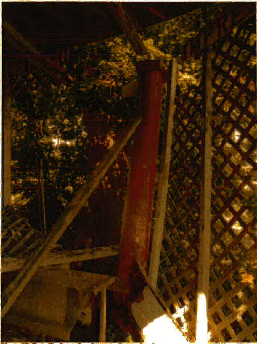
Photo #5: Detached porch column and rotted rafters.
