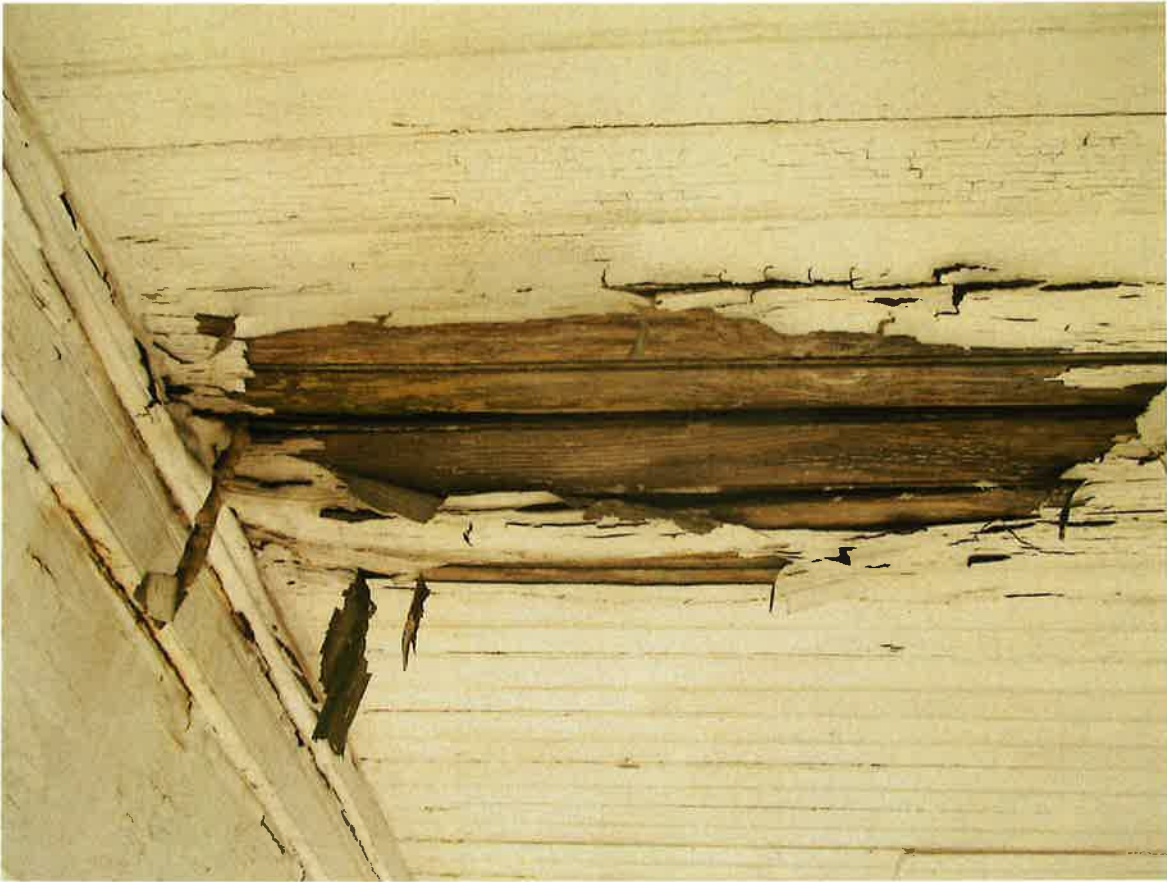
Photo #1: Ceiling damage at exterior porch.
