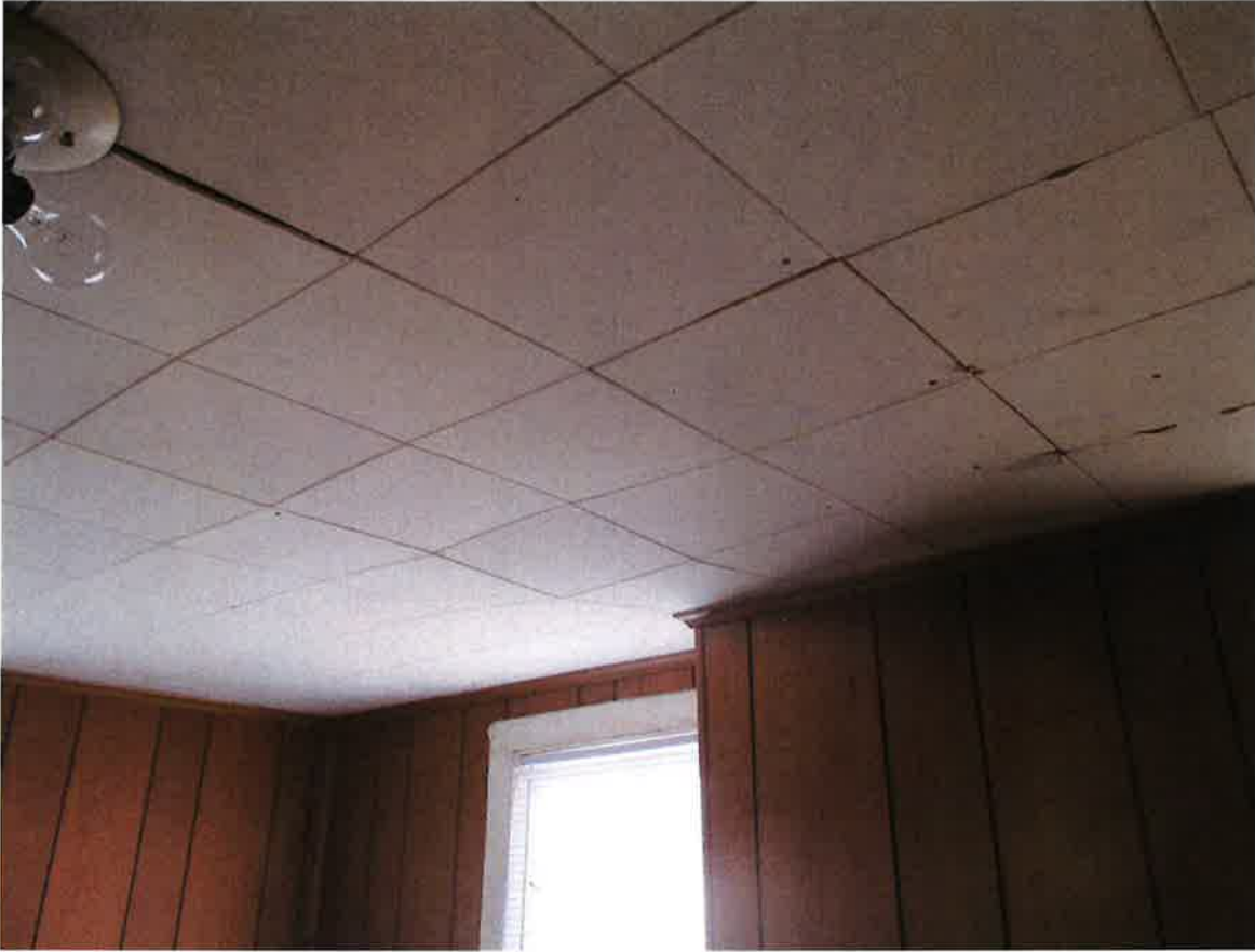
Photo #5: Large deflection is present in first floor ceiling at front left office.
