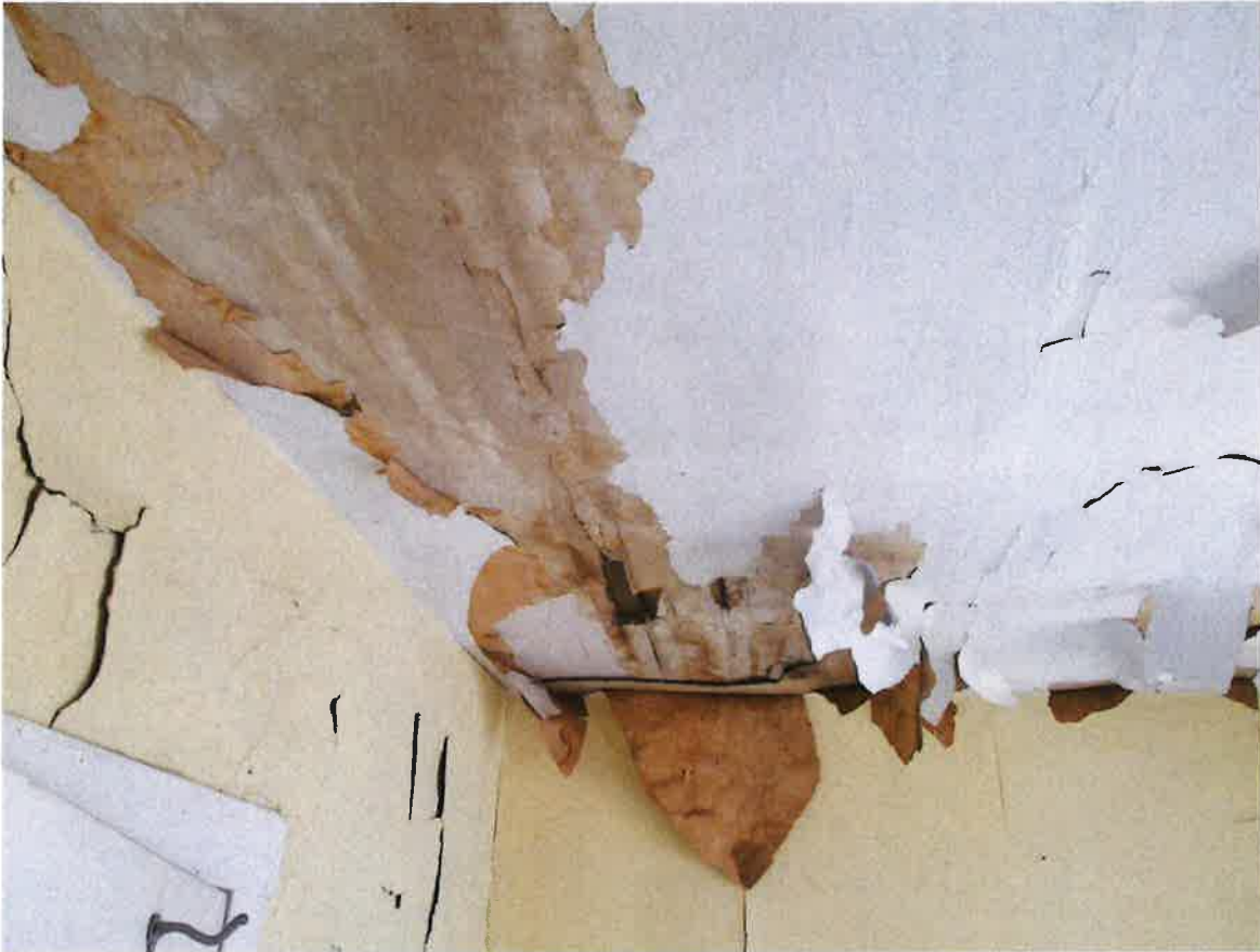
Photo #9: Water damaged and bowed plaster ceiling.
