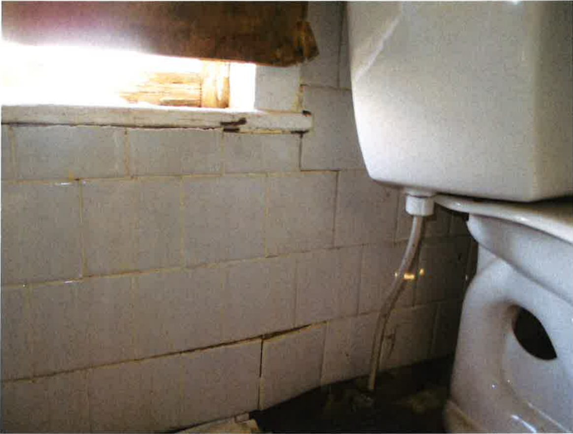
Photo #6: Cracked and bowed wall tile at rear bathroom.
