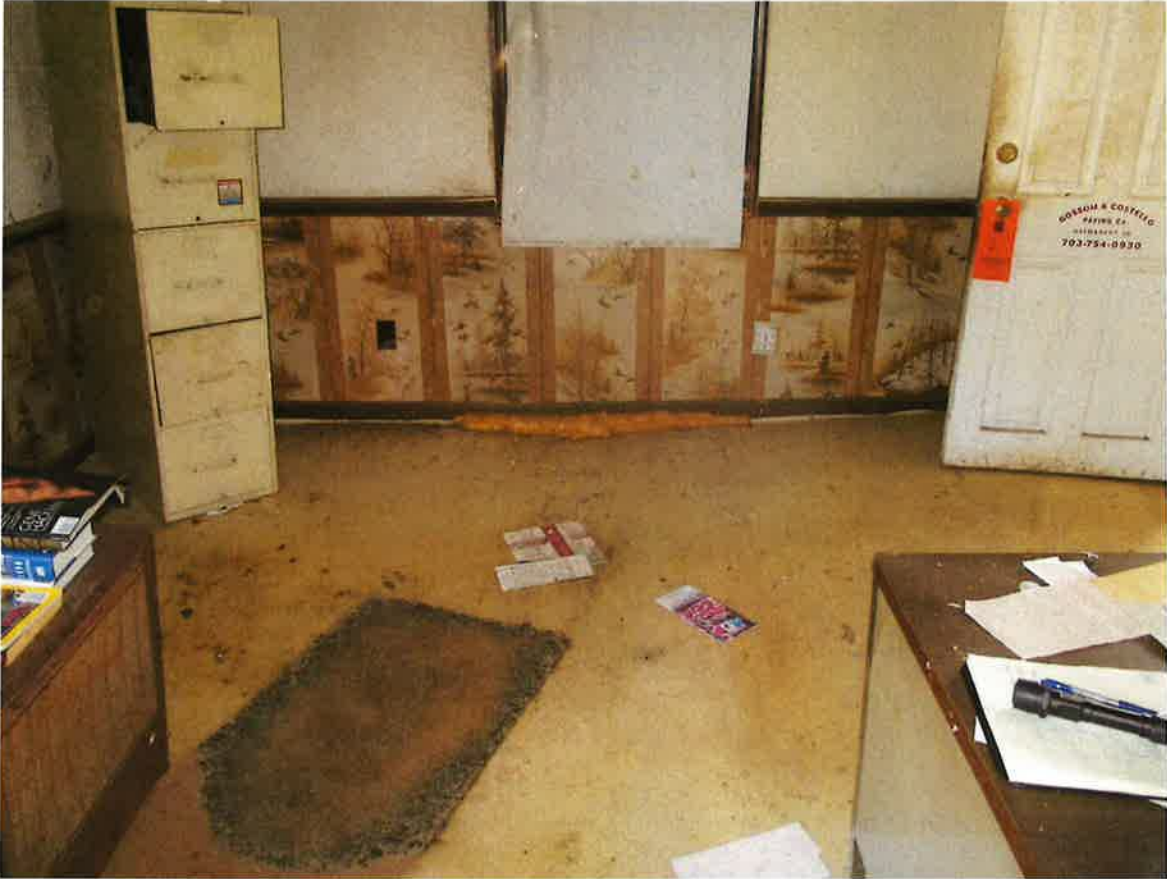
Photo #4: Severe bow is present in floor at interior of the house with insulation filling the void.
