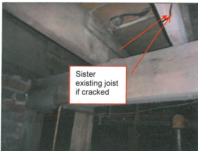
Photo 2 – View of joists with possible crack where indicated
