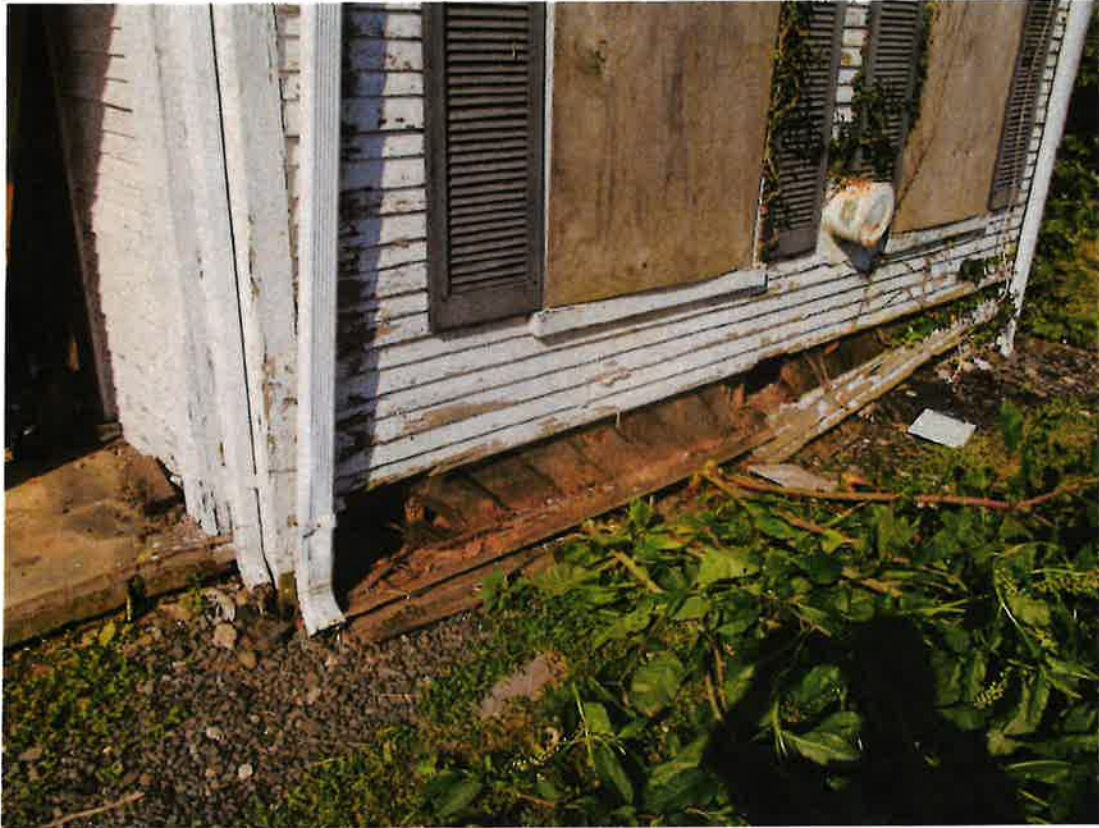
Photo #4: Collapsed siding board at base of wall.
