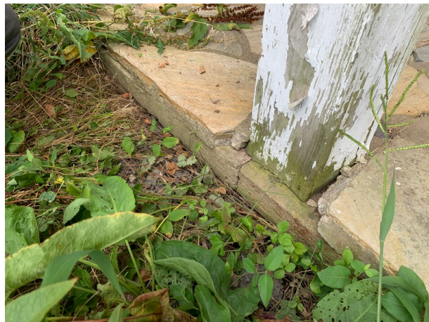
Wood Rot on Concrete
