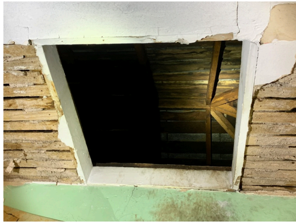
Spaces in Wood Roof Paneling from Attic
