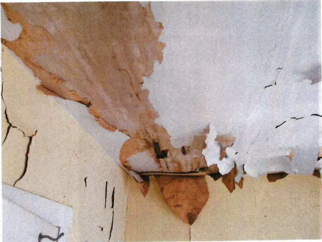
Photo #9: Water damaged and bowed plaster ceiling.
