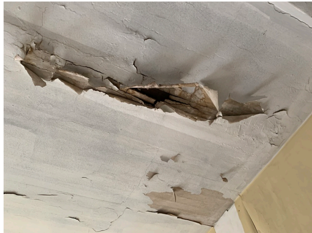
Ceiling condition with peeling paint and cracking
