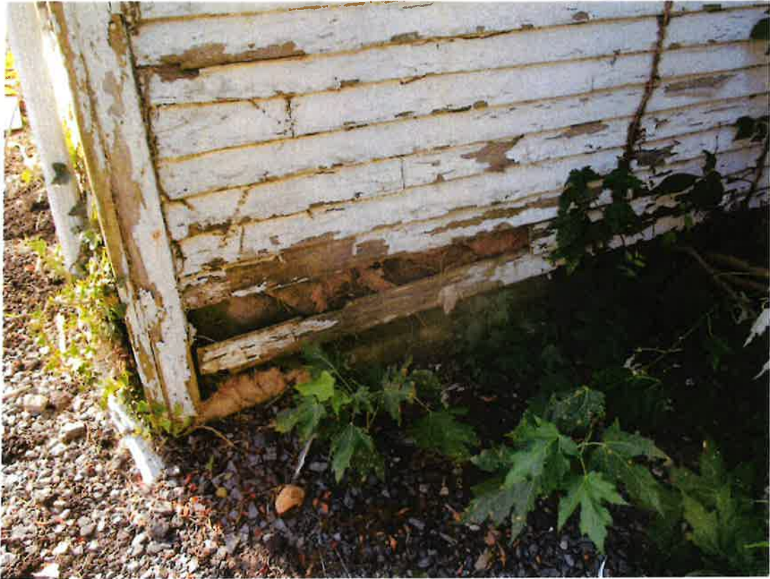
Photo #8: Rotted and missing sheathing boards.
