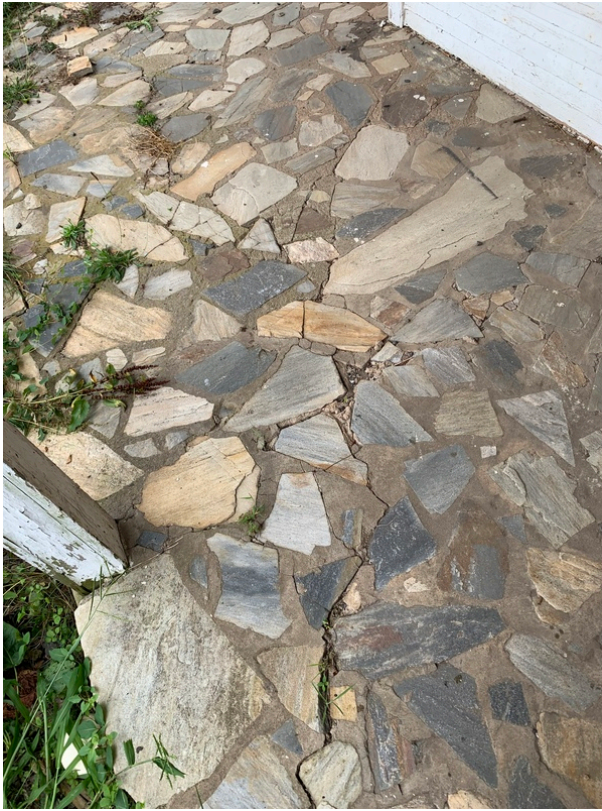
Cracking of Concrete of Stone Porch
