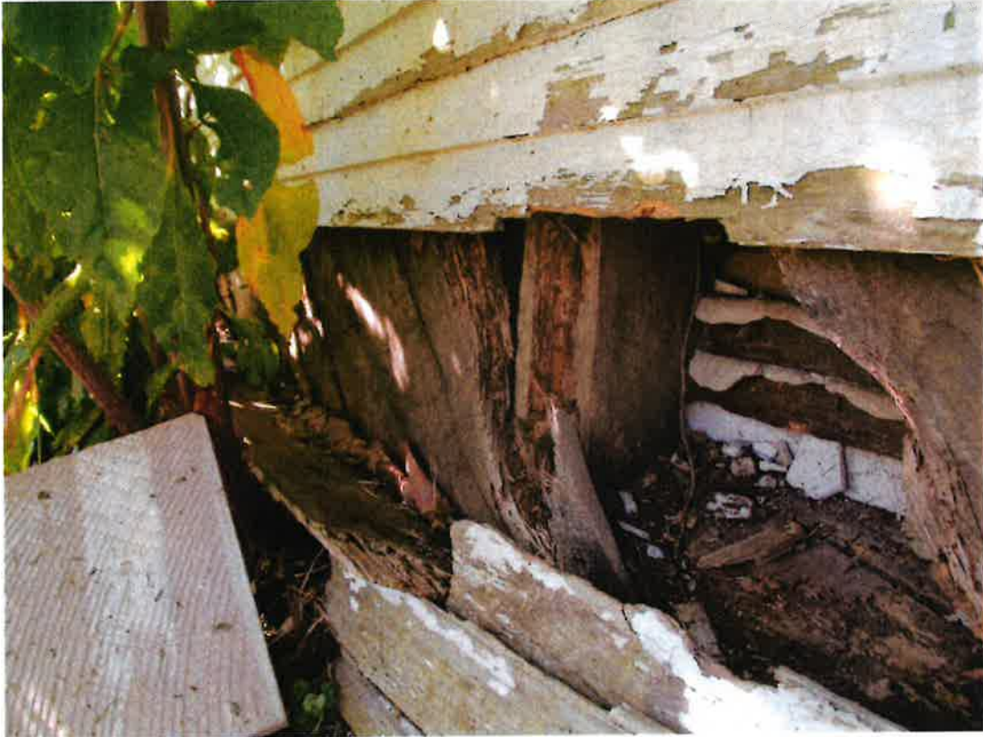
Photo #5: Exterior exposed and rotted wood studs, diagonal brace and sill plate.
