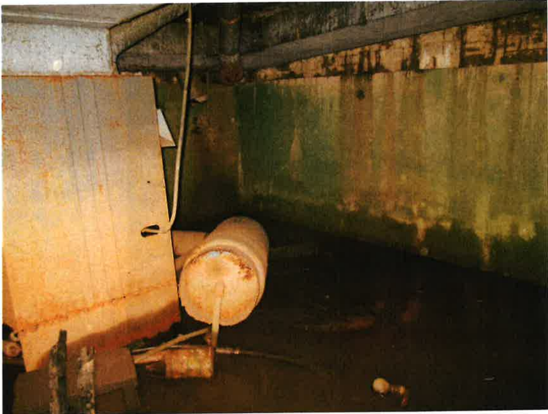
Photo #11: Standing water throughout basement level.
