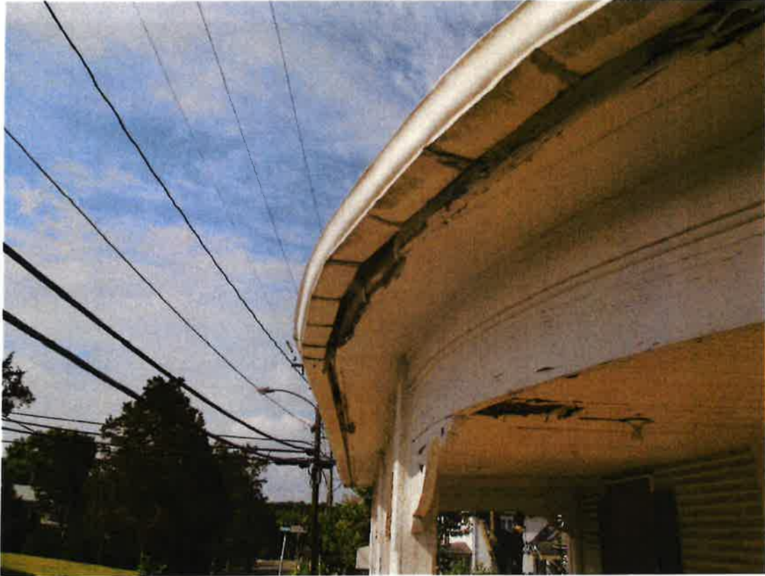
Photo #2: Soffit damage at edge of porch gutter.
