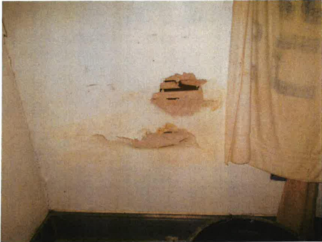
Photo #12: Plaster damage on face of wall.
