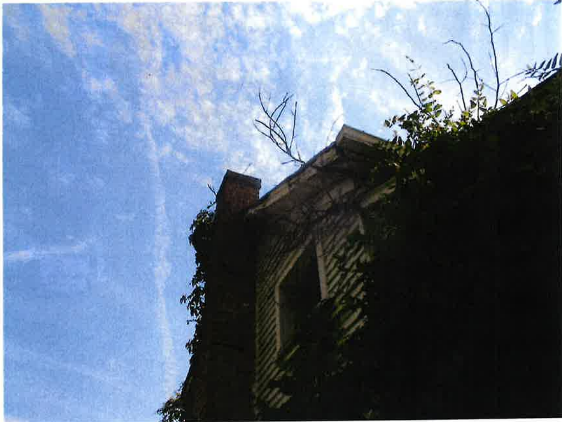
Photo #7: Rotted rake board.
