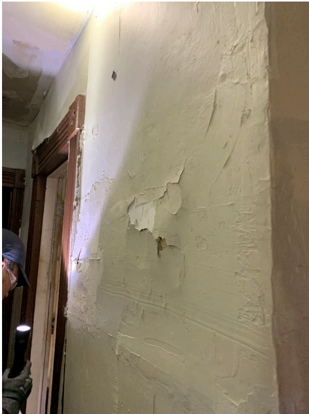
Typical wall condition with peeling paint and cracking
