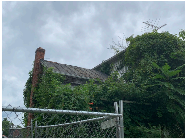
Addition roof (upper) of metal standing seam with mudroom roof of shingles (lower)
