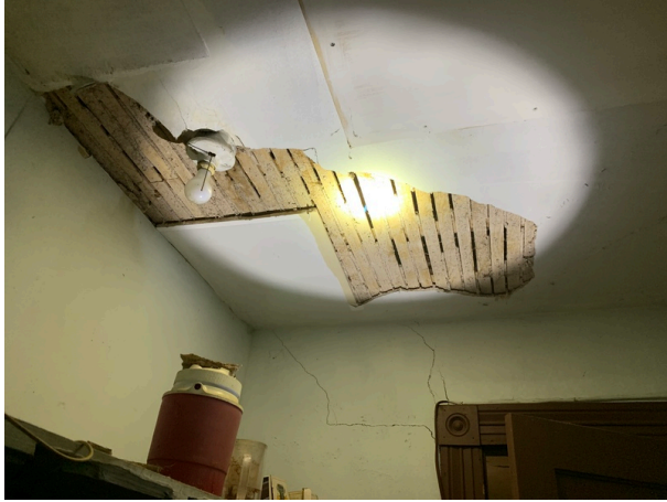
Collapsed ceiling finishes
