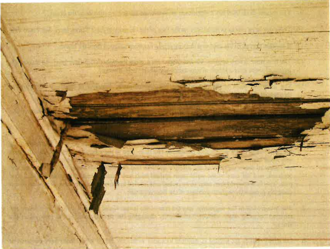
Photo #1: Ceiling damage at exterior porch.
