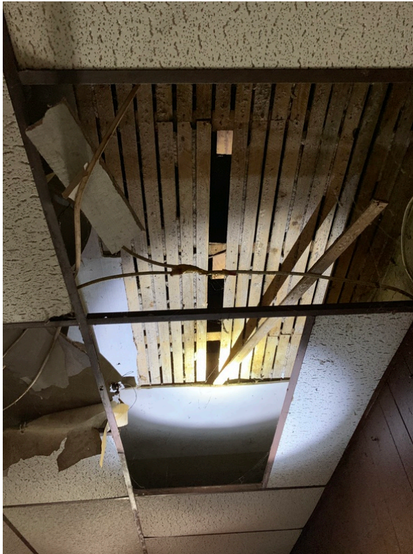
Collapsed ceiling finishes
