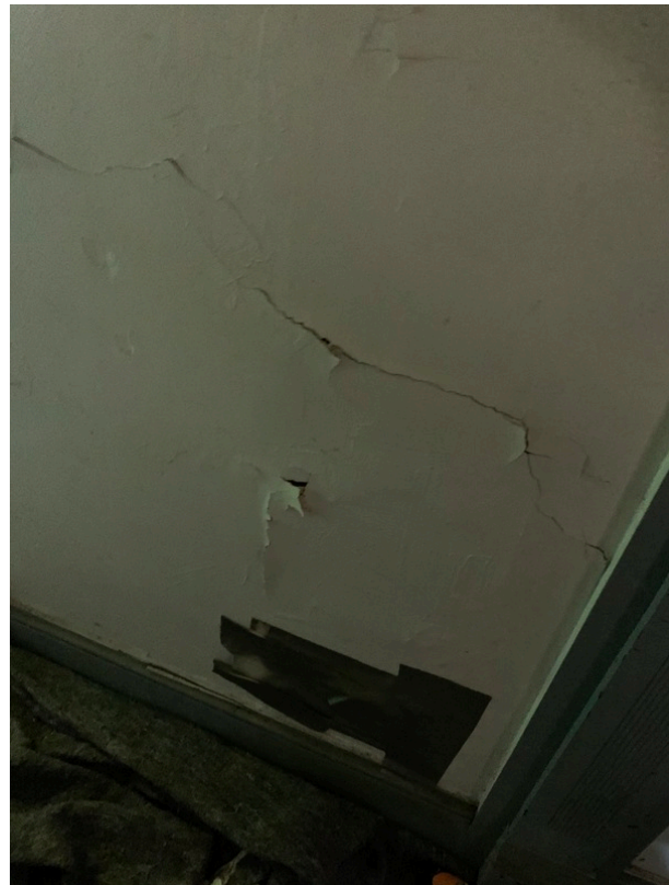
Cracks along Wall
