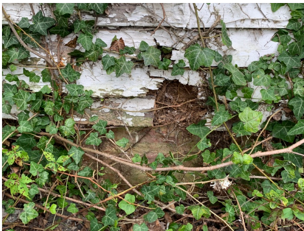
Close up of siding which growth has severely damaged
