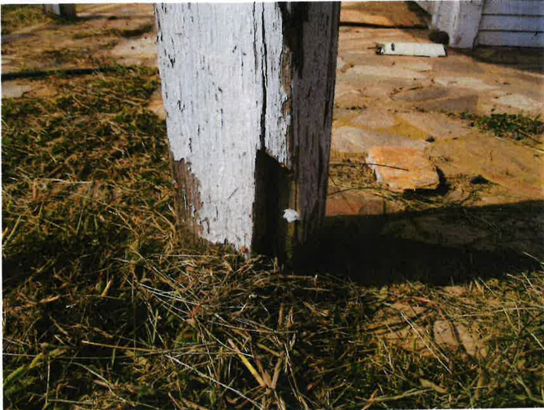
Photo #3: Rot at base of porch post.
