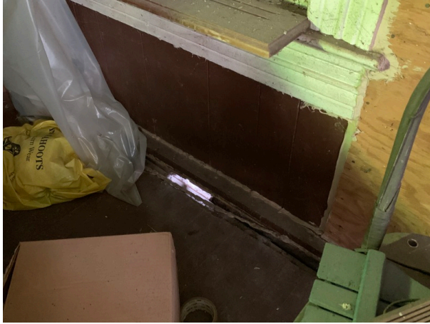
Hole in bottom of Wall in Kitchen, goes to the outside
