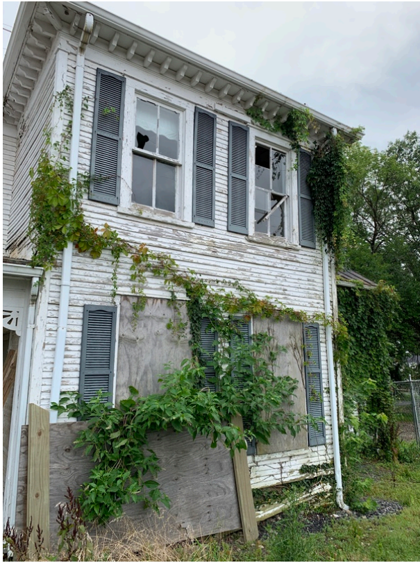
Organic Growth on North Exterior
