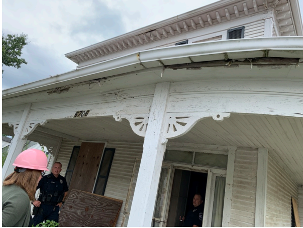
Wood Rot under Roof
