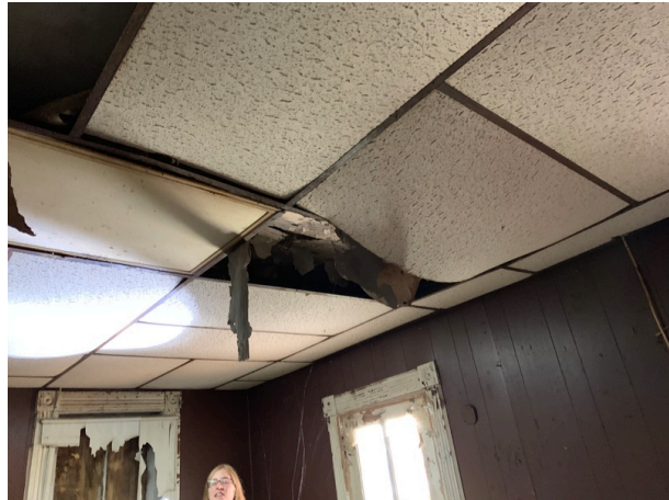
Collapsed ceiling finishes
