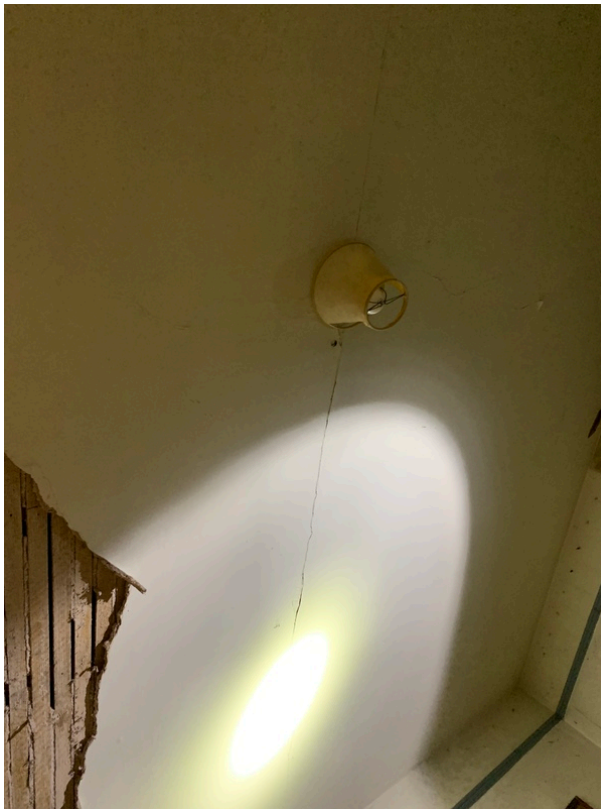
Crack in Ceiling of 1st Floor
