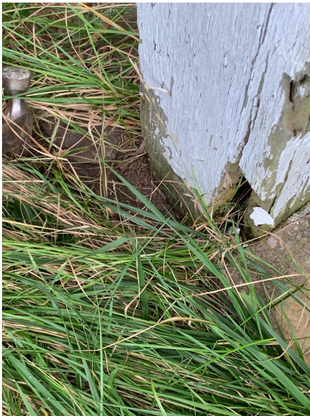
Wood Rot of Support on Earth
