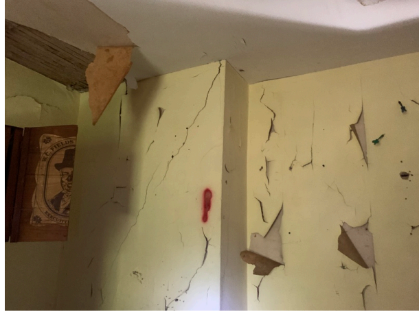
Typical wall condition with peeling paint and cracking
