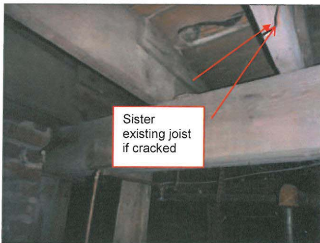
Photo 2 – View of joists with possible crack where indicated
