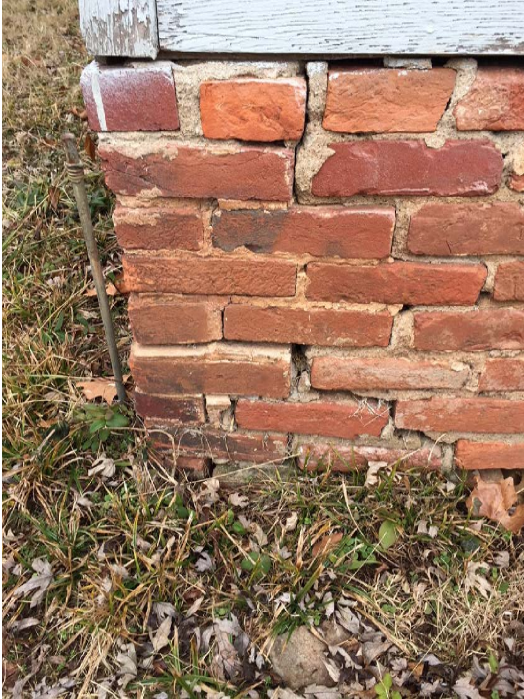
PHOTO # 1: Foundation Deterioration
