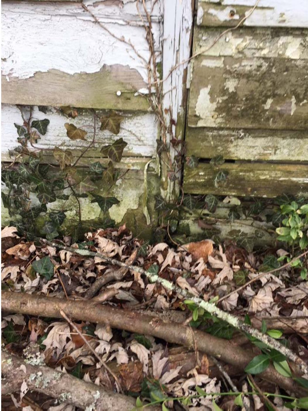
PHOTO # 3: Wood Framing in Contact With Soil
