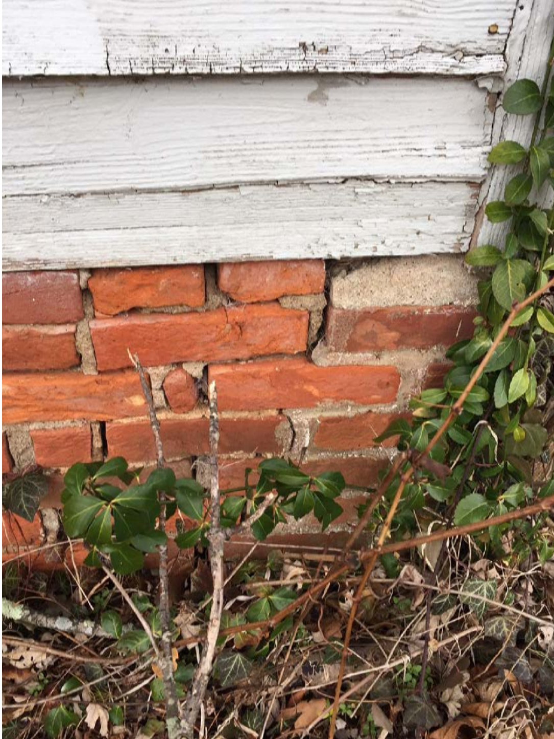
PHOTO # 2: Foundation Failure and Deterioration
