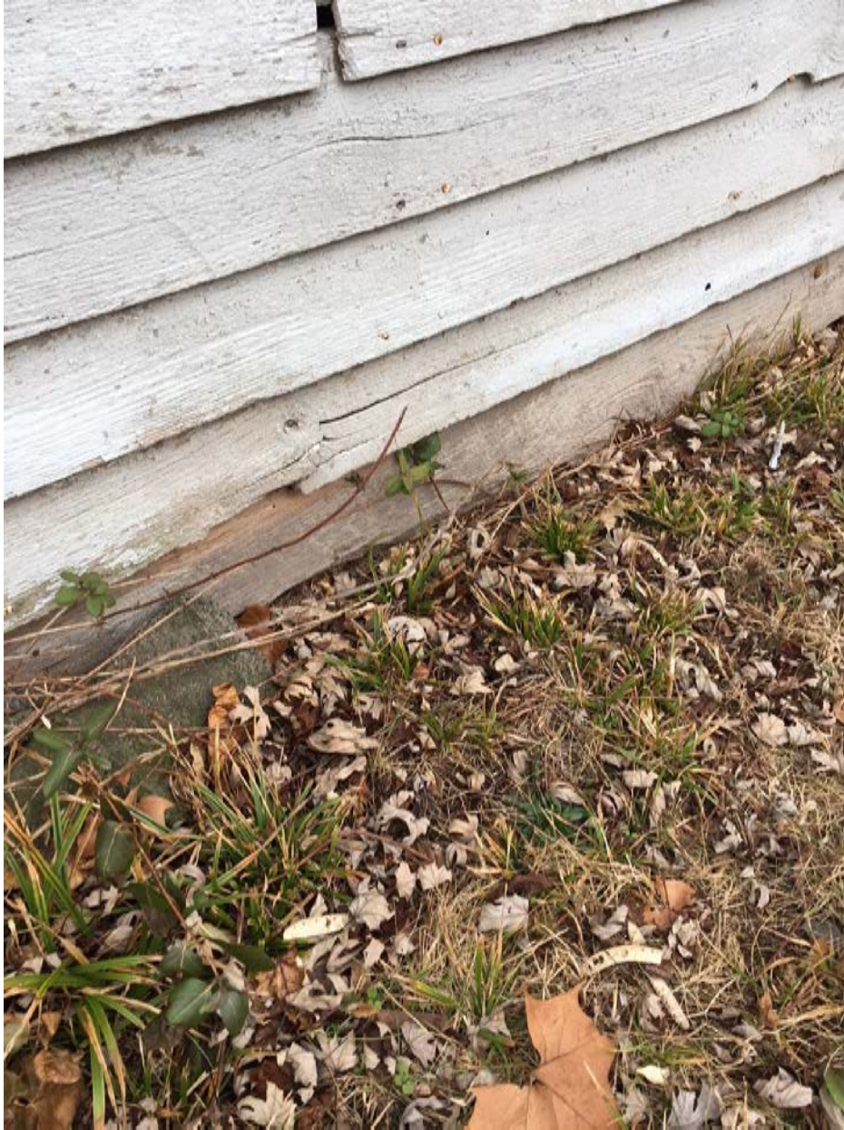
PHOTO # 4: Wood Framing in Contact With Soil
