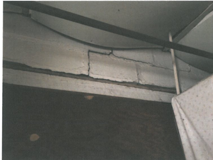
Photo 5 – masonry failure between Area A and B
