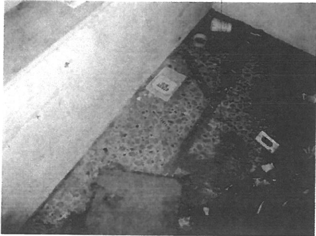
Photograph 1 A view of the linoleum in the small 1 st floor office in the main entry bay. There are two layers of asbestos linoleum as well as an underlying layer of black mastic/glue which is also asbestos containing.
