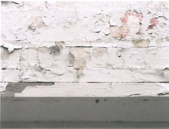
Photo 22 – Wood plate no apparent lintel
