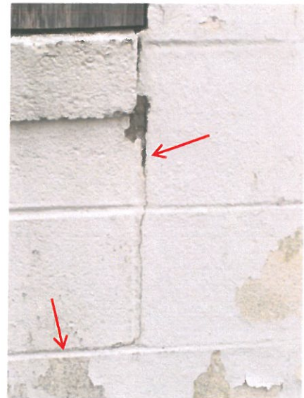
Photo 19 – Early signs of stress
