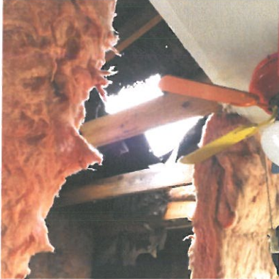
Photo 2 – Hole in roof
