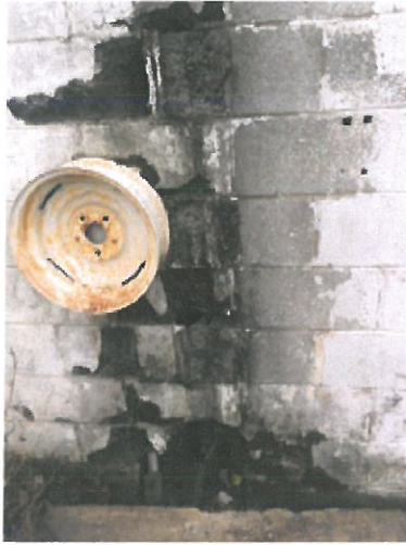
Photo 10 – Deteriorated exterior wall
