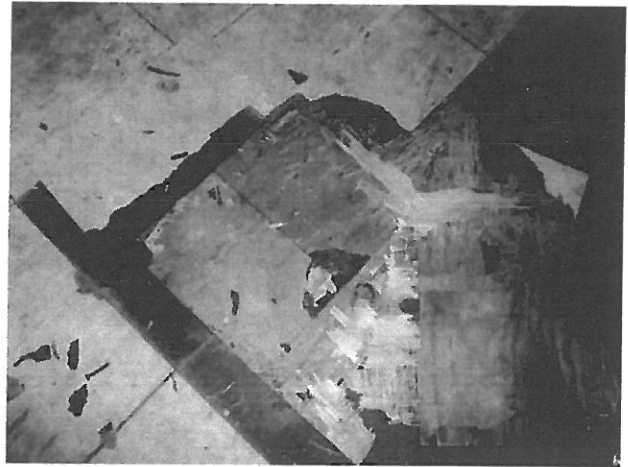
Photograph 2 View of the flooring system on the 2 nd floor. The grey 12" tiles and associated mastic are asbestos containing and affixed to a plywood subfloor. Underneath the plywood are asbestos containing 9" floor tiles and mastic which are also applied to a wooden floor. These 9" tiles/mastic can also be expected to be located underneath any erected walls.
