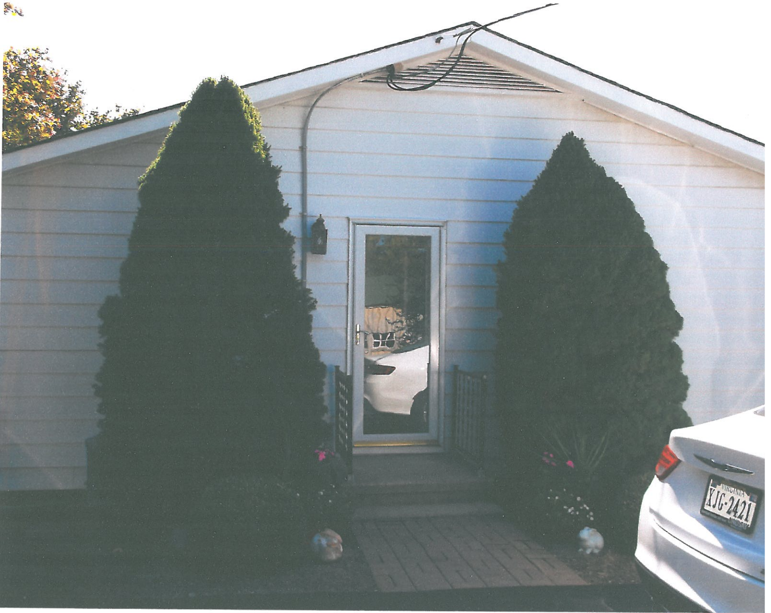
Attachment: 6705 Madison Street - Replace Roof- Paint Shutters & House (2556 : 6705 Madison Street - Roof Replacement & Additional Work)
