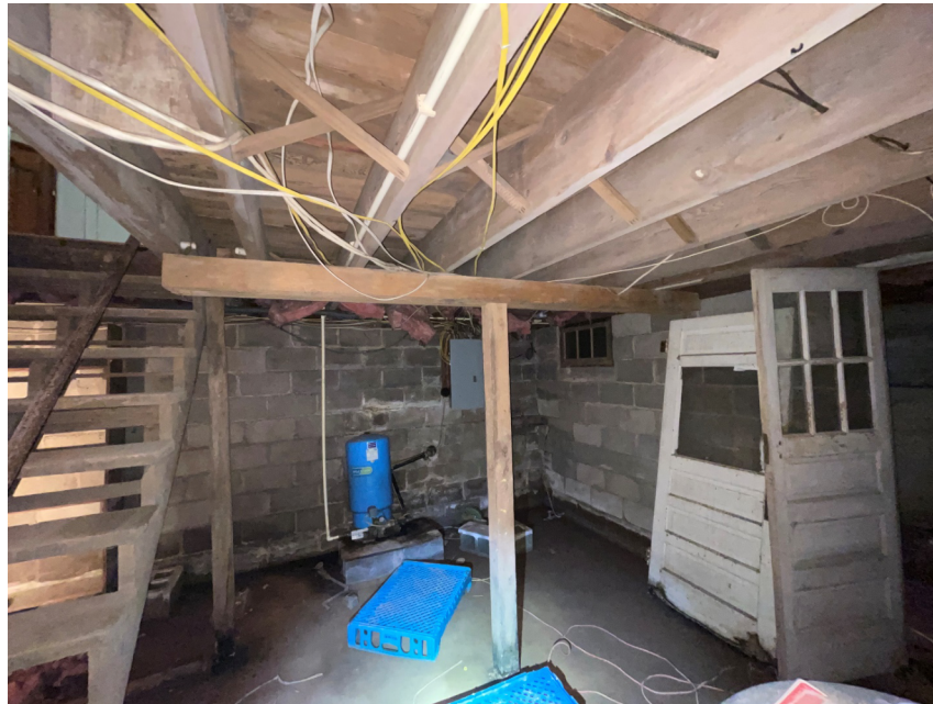
Basement Observation #9 (Photo 2 of 3)
