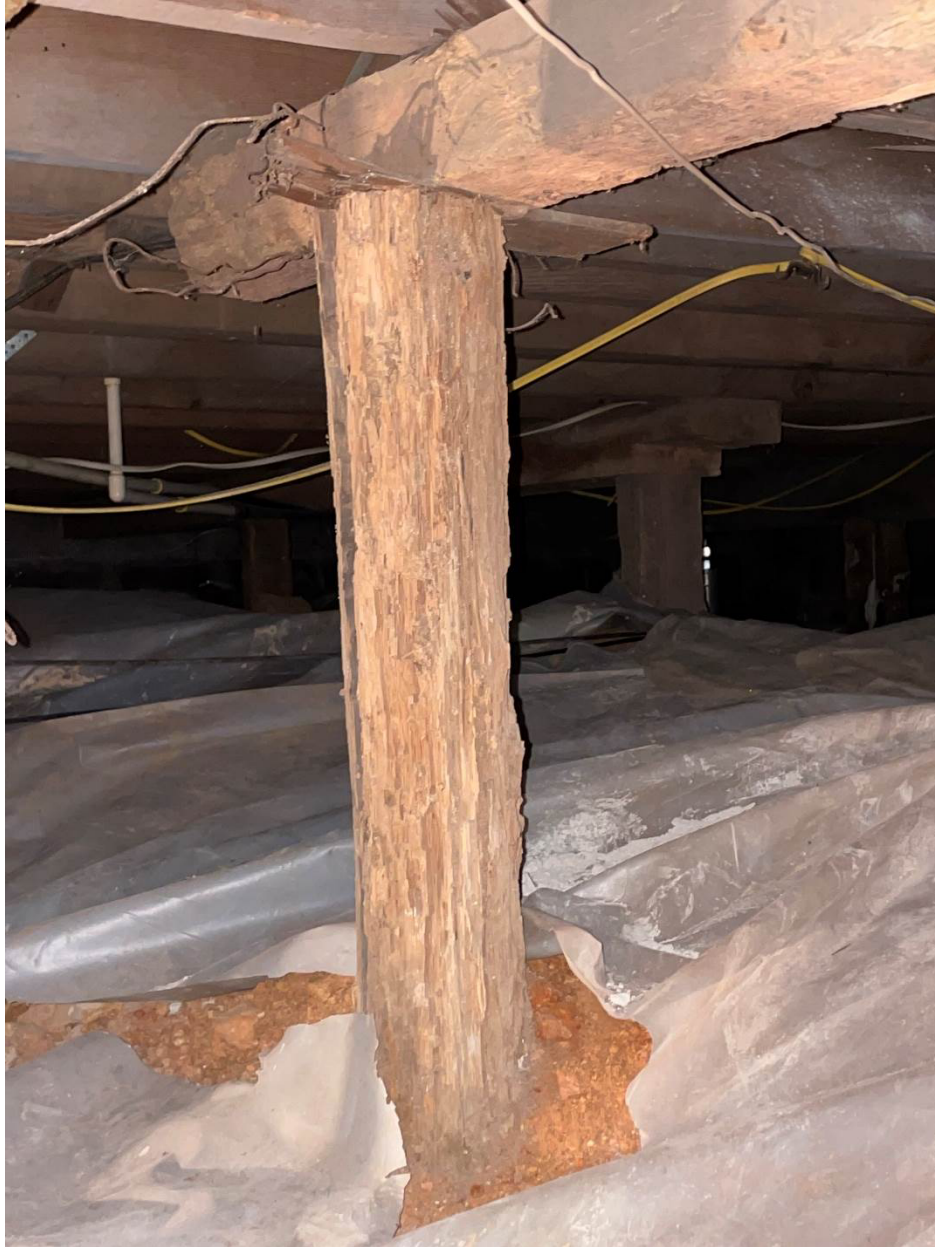
Basement Observation #9 (Photo 3 of 3)
