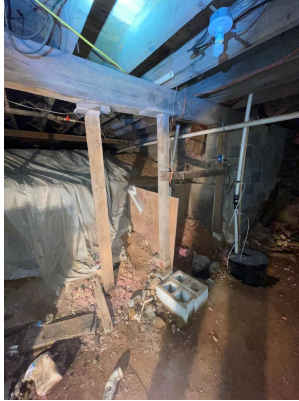
Basement Observation #9 (Photo 1 of 3)
