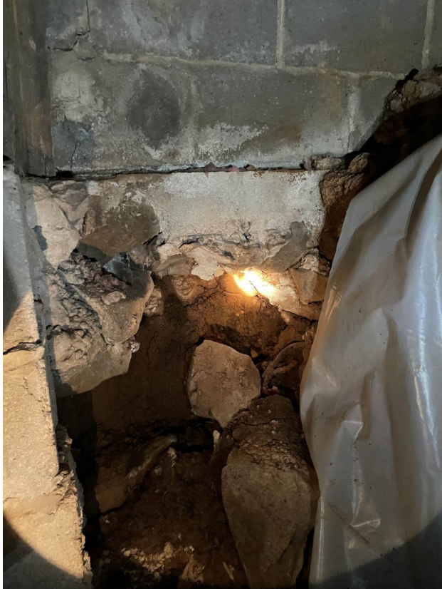
Basement Observation #4 (Photo 1 of 2)
