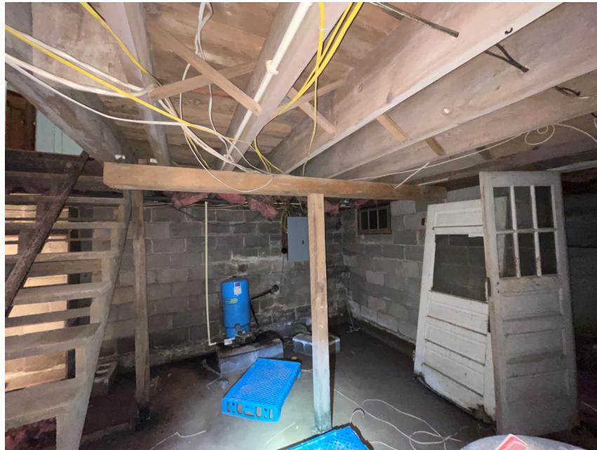
Basement Observation #9 (Photo 2 of 3)
