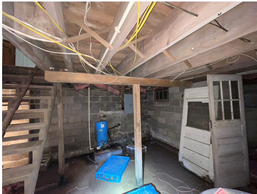
Basement Observation #9 (Photo 2 of 3)
