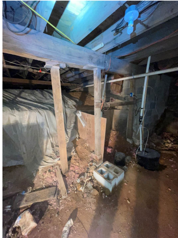
Basement Observation #9 (Photo 1 of 3)
