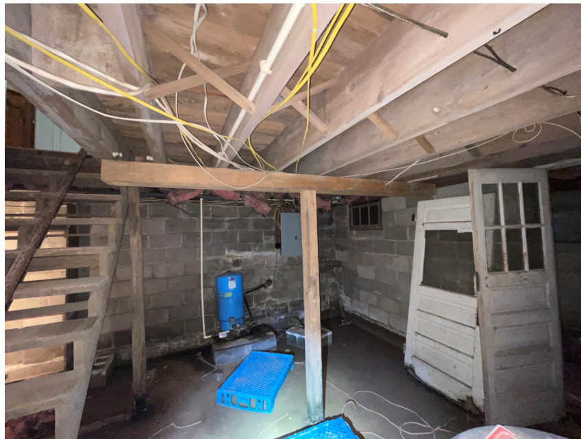
Basement Observation #9 (Photo 2 of 3)
