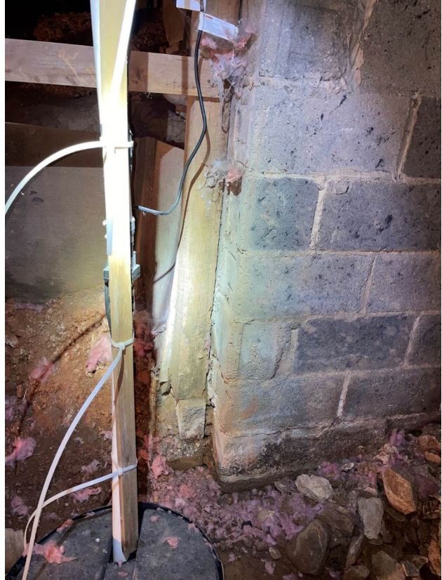
Basement Observation #4 (Photo 2 of 2)
