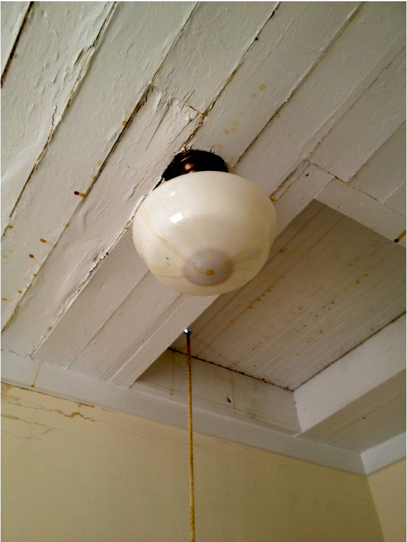
Rust colored drips suspected to indicate wood rot. Water saturated and split walls, warped ceiling strips, and collected in (non-functioning) ceiling fixtures.
