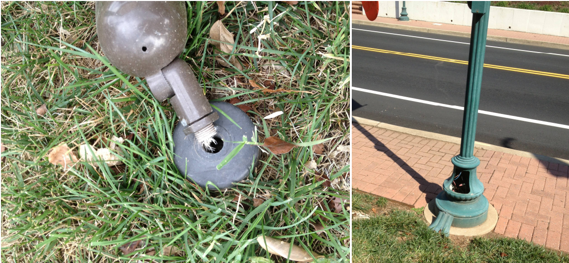
Signage light severed (presently stored inside museum). Exposed wiring in pedestal of street light, near entrance steps.
