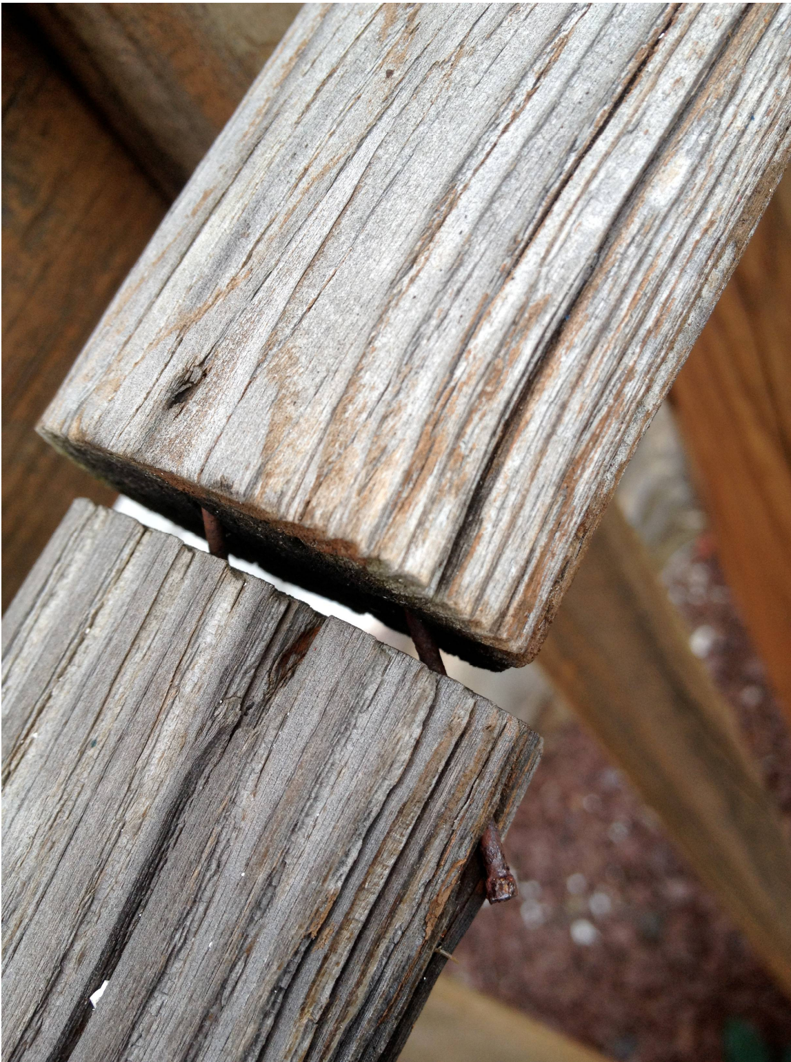
Exposed rusty nails, splintering, vegetation growing over ramp.
