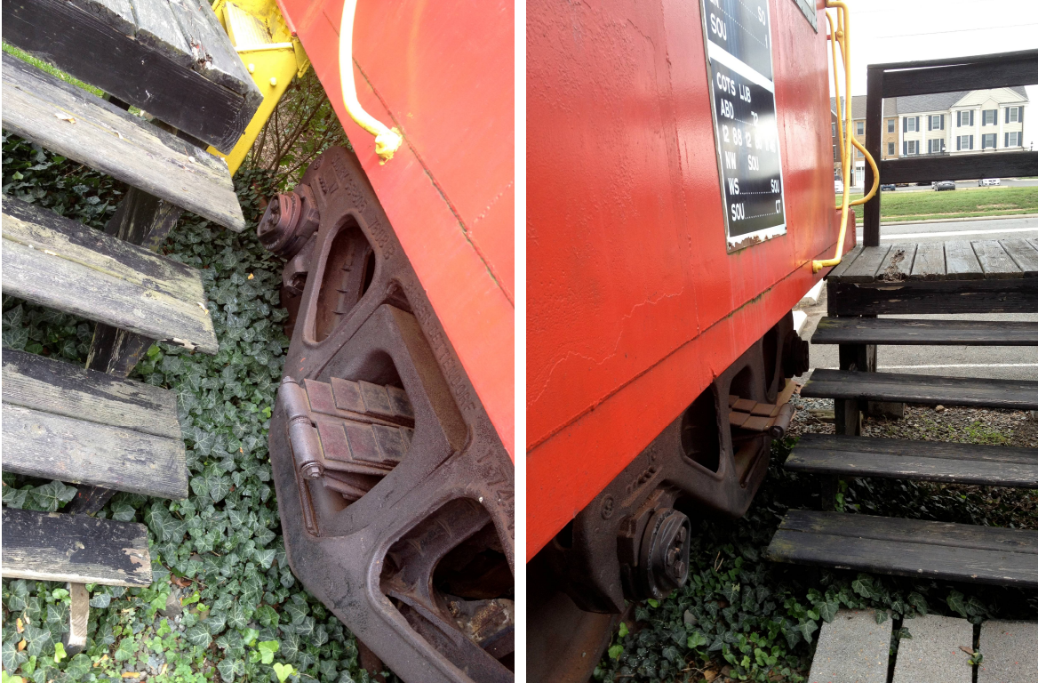
Missing step, no protection to prevent from severe injury between steps and steel.
