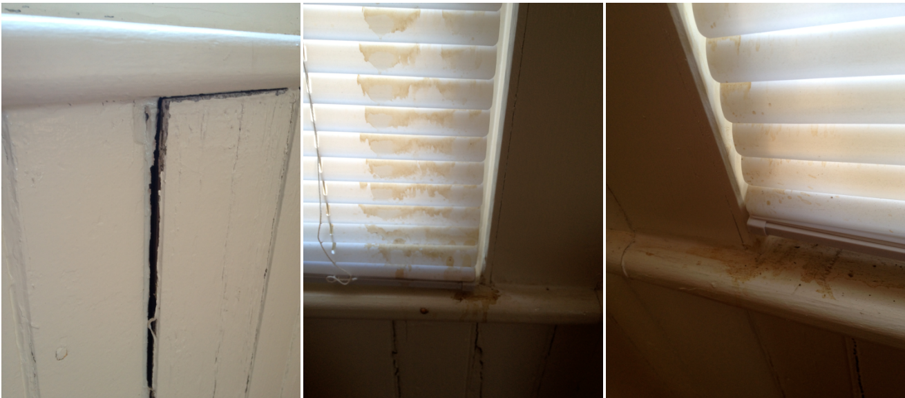
Example of many areas of buckled wainscoting on 1 st floor. Water pooled in Venetian blind housing and poured down the walls.
