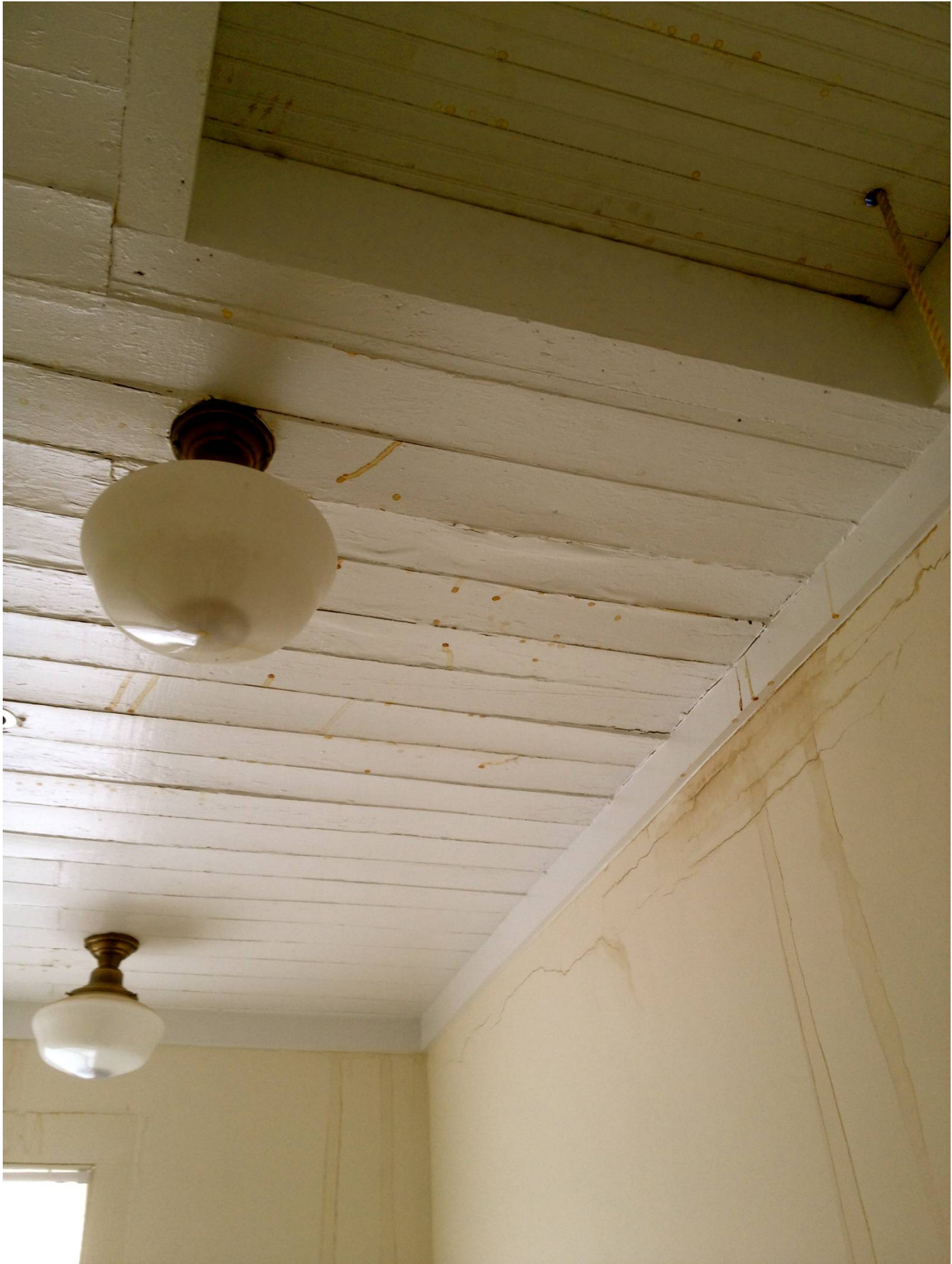
Attachment: Photos of Hurricane Sandy Damage @ Museum (1257 : Museum Report)
