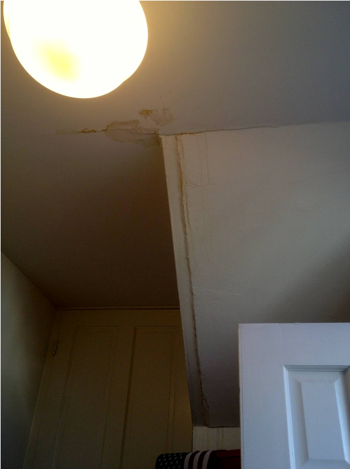
1 st floor entryway, water intrusion into light fixture, cracks, stairway above. Water stains rust-colored, suspected to be from wood rot.
