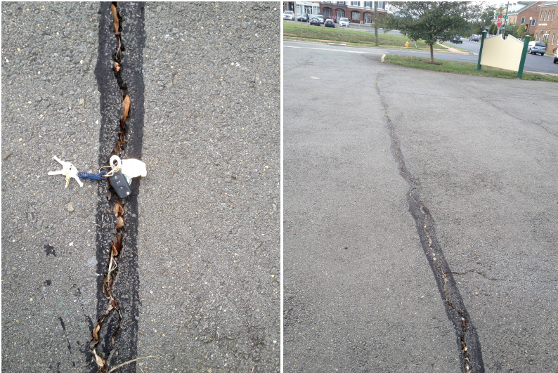
Parking lot. Crack allows for ice, worsening of expansion, and eventual upheaval.
