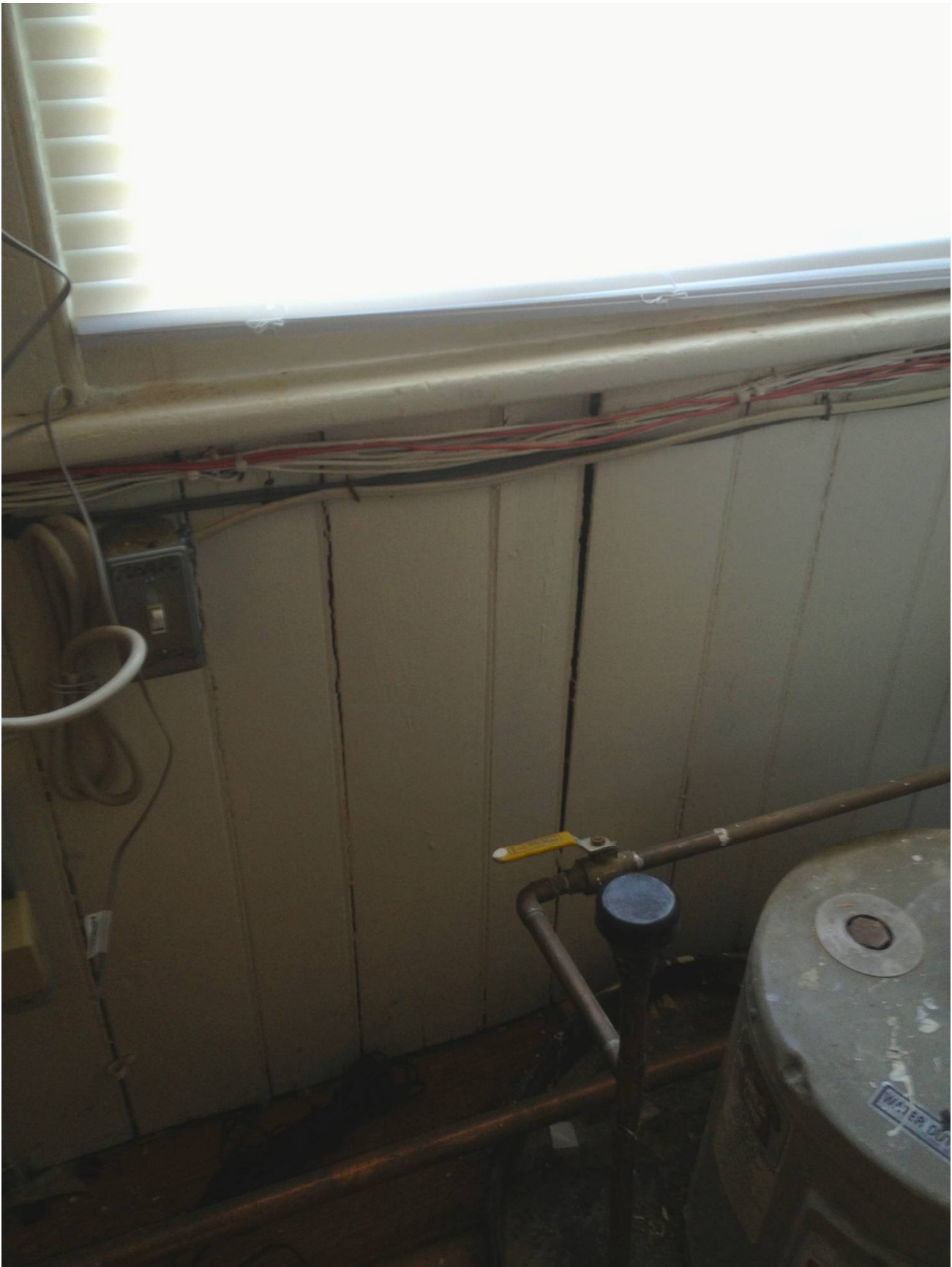
Water damaged, buckled and split wainscoting in electrical room.
